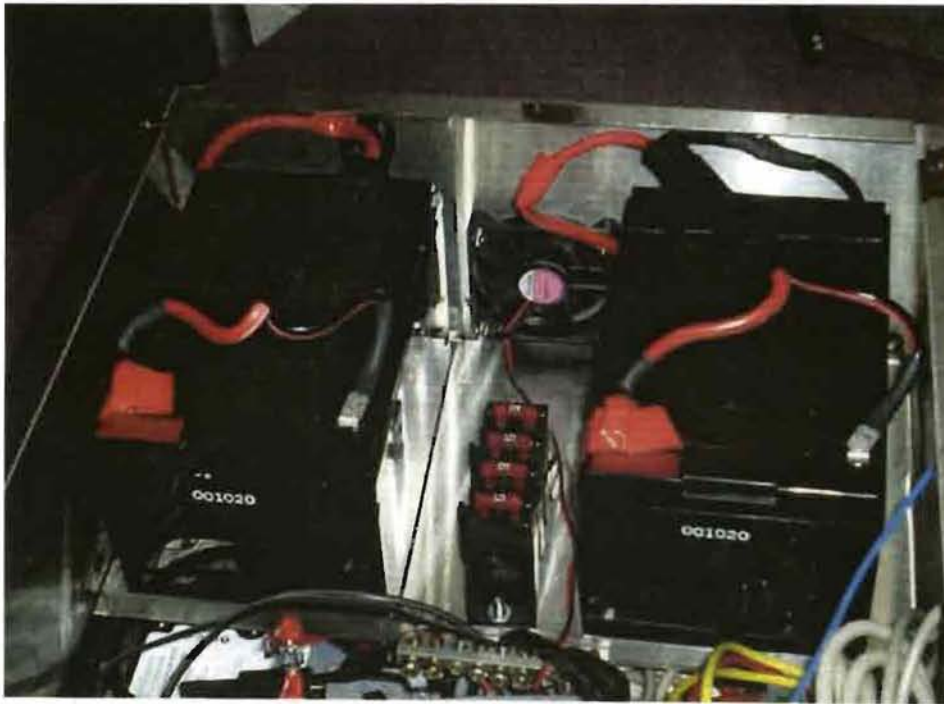
Figure 5: Batteries, fuse block, and ground bus bar.
