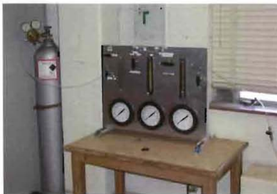
Figure 11: Dry air cylinder and flow panel
