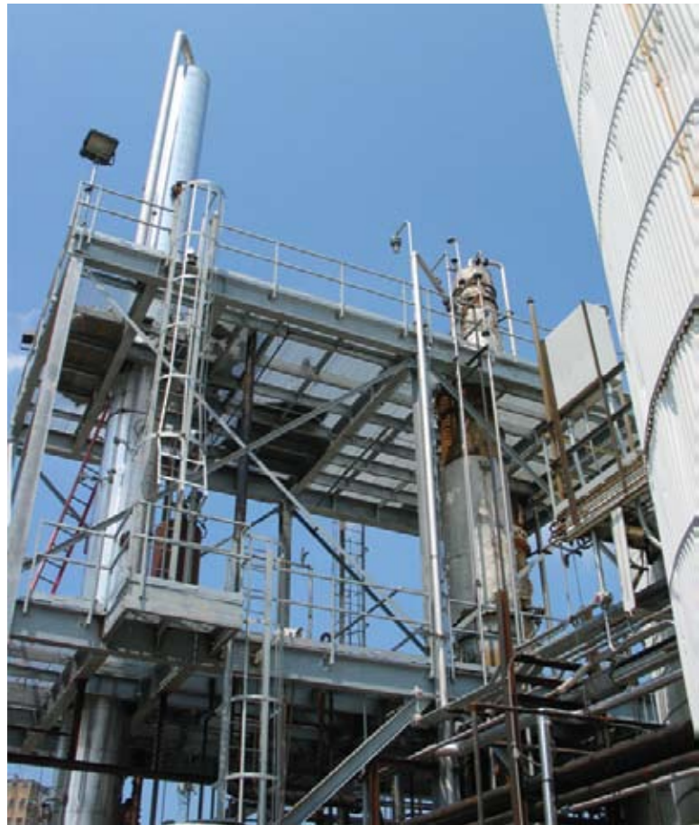
Biodiesel production facility. Credit: Kelly Tiller, University of Tennessee
