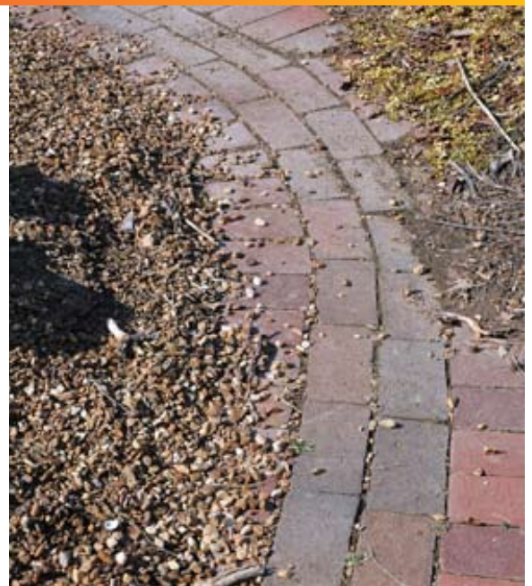
Lack of edging creates a poor division of elements.
