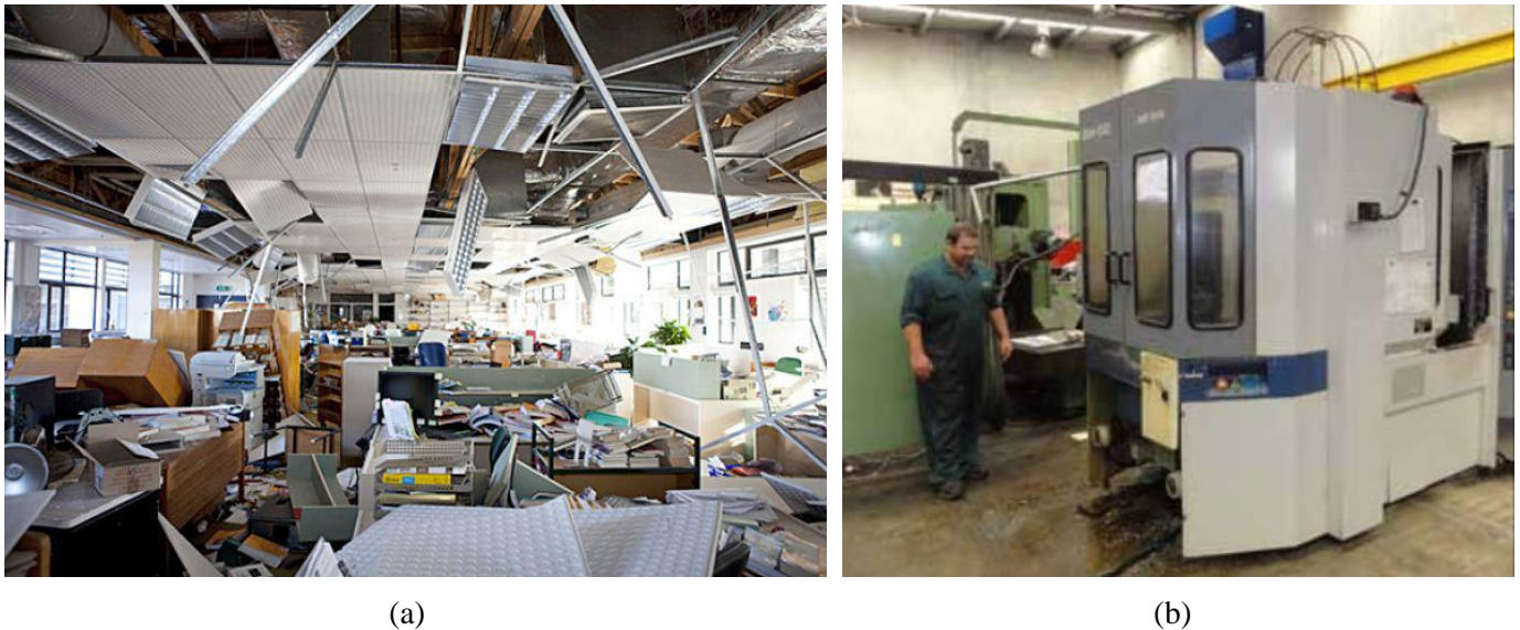
Fig. 1. Examples of damage to building contents: a) commercial environment (NIWA [20]), and b) displacement of heavy equipment in an industrial facility [19].
