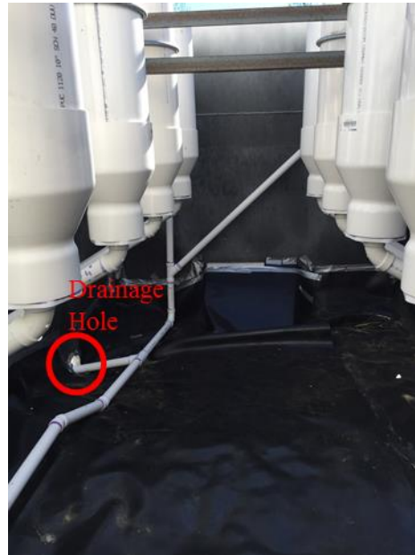
Figure 6.5: Installation of a drainage system using 1.5” diameter PVC pipes, 2 wyes, 22.5, 45, and 90 degree elbows, and one tee.
