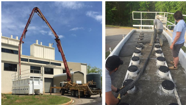
Figure 6.8: Backfilling the test bed, on the left utilizing a pump truck and on the right with a line pump.
