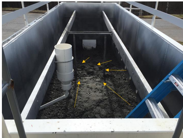
Figure 6.4: Gravel graded to promote drainage to the hole on the left side of the tank.
