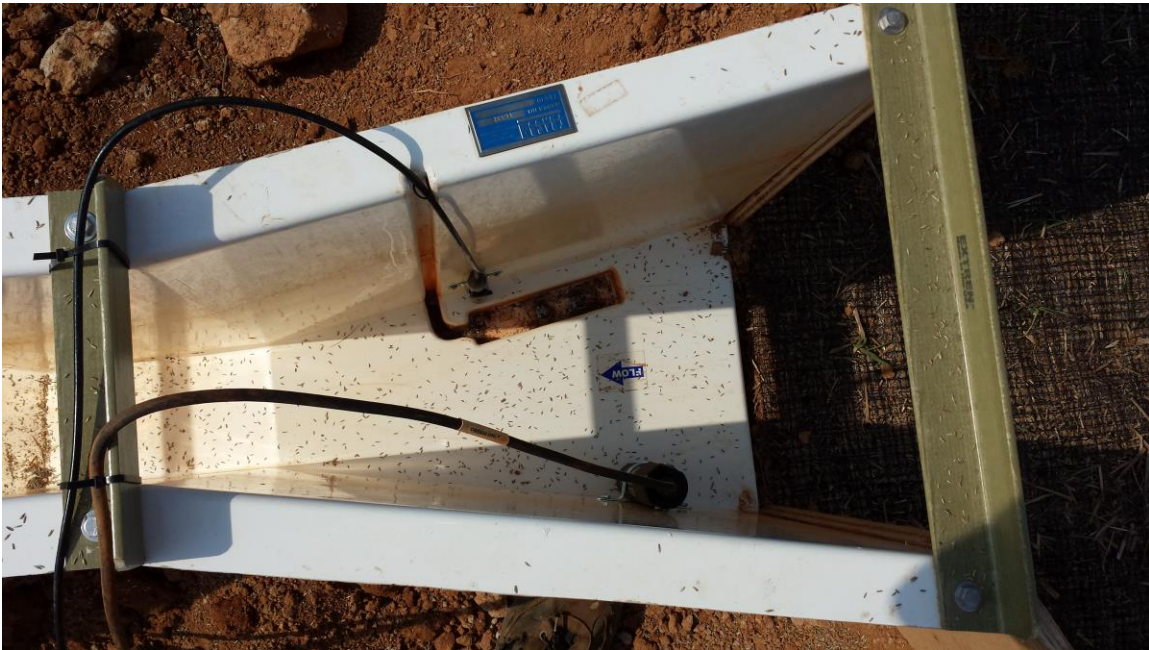
Figure 5.4: Probes mounted in the Parshall flume.
