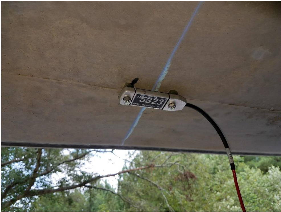
Figure 73: Close-up of NEXT D BDI Strain Gauge
