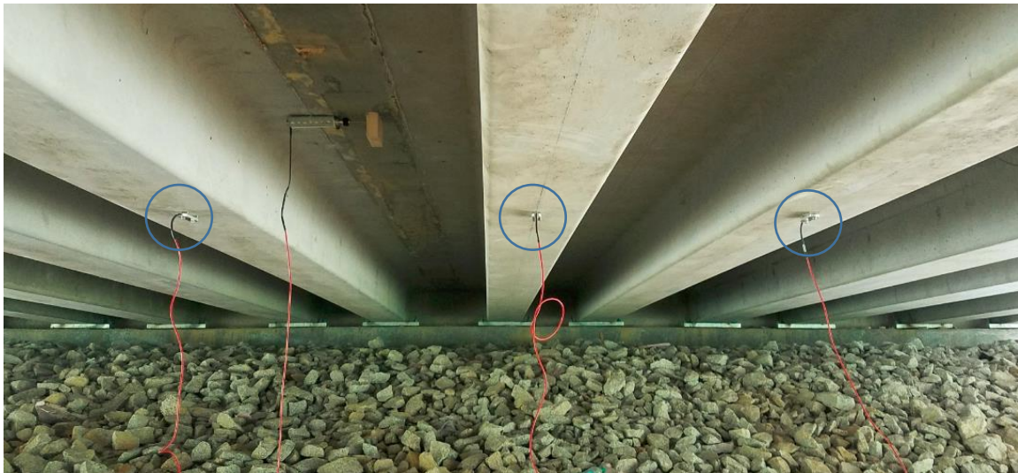
Figure 72: BDI Strain Gauges on NEXT D Span
