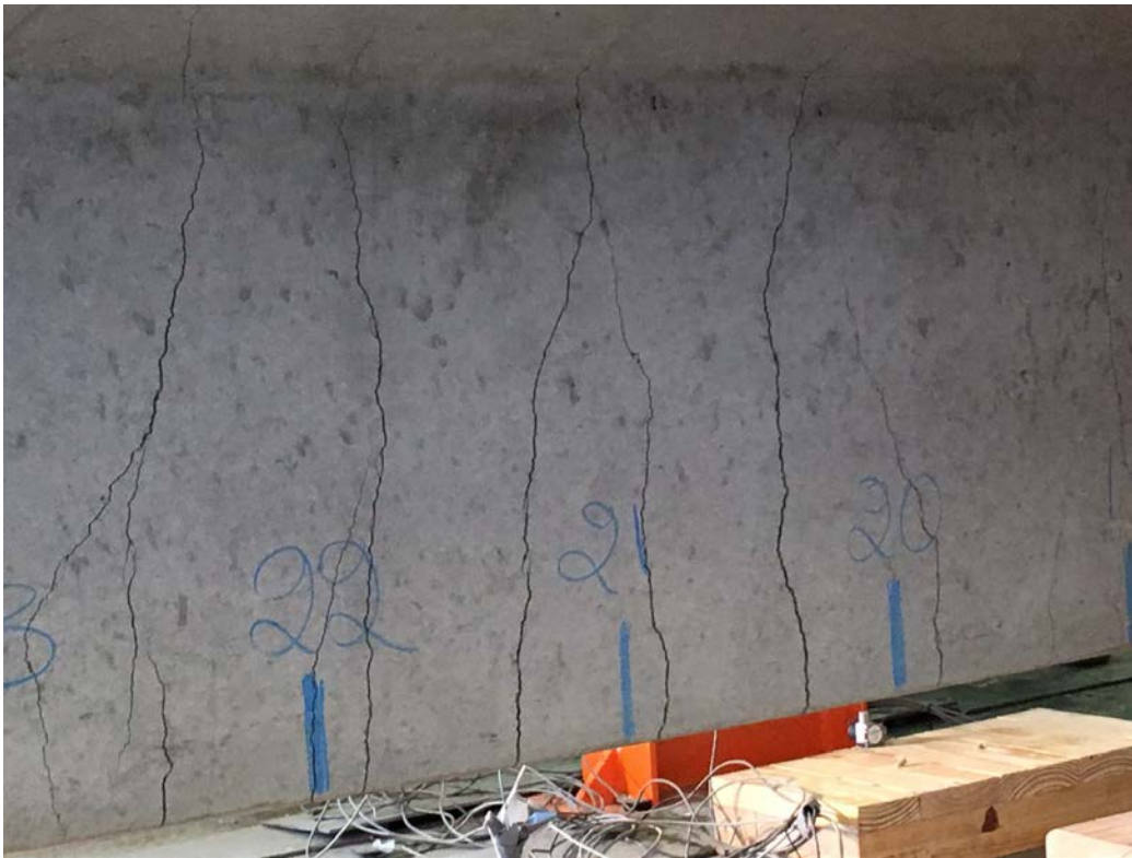
Figure 31. Widening of the cracks and formation of new cracks during flexural load test
