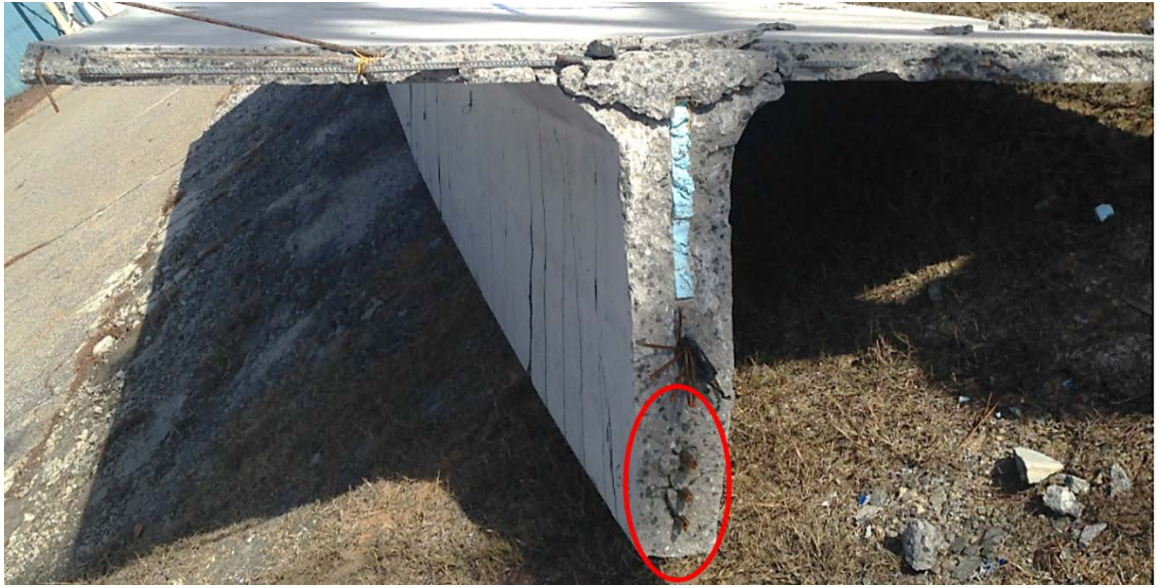
Figure 35. Specimen L1 at location of strand rupture
