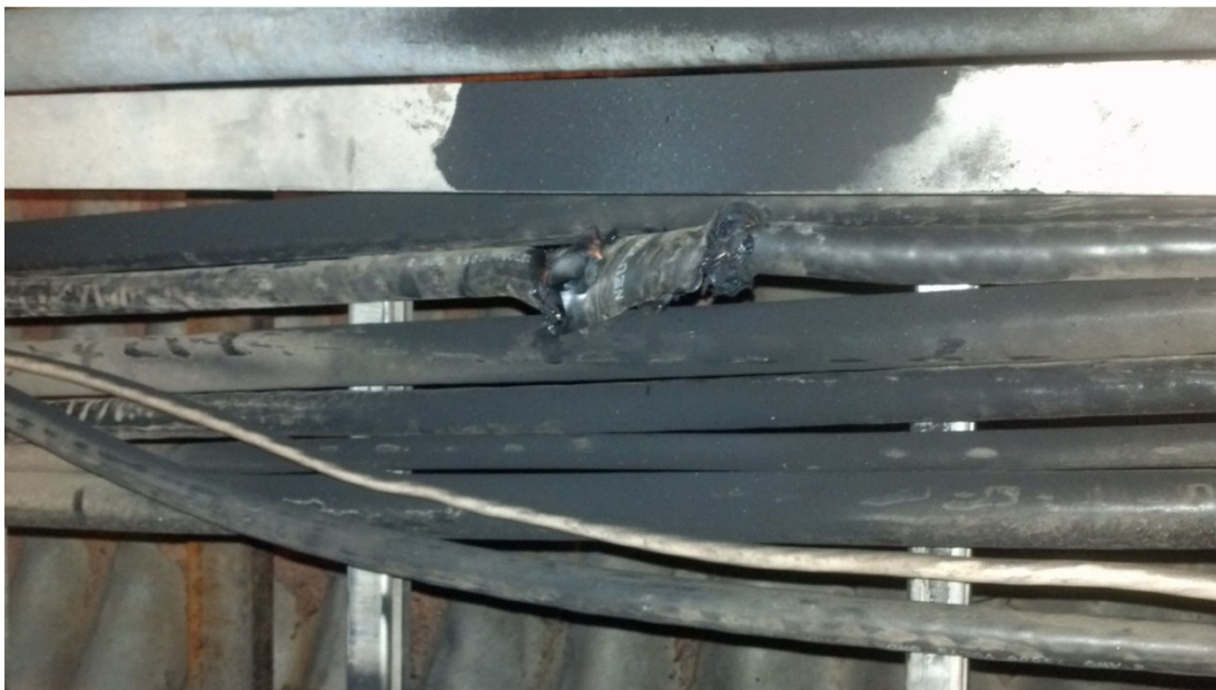
Figure 1: Water-Tree Fault in Old Cables
