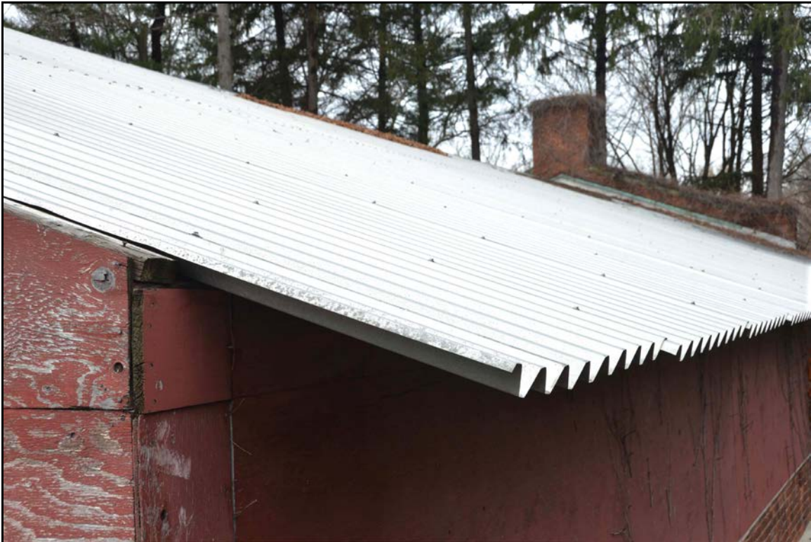
Figure 4.34: Detail illustrating condition of corrugated aluminum roofing, 2016 (Photograph by author).
