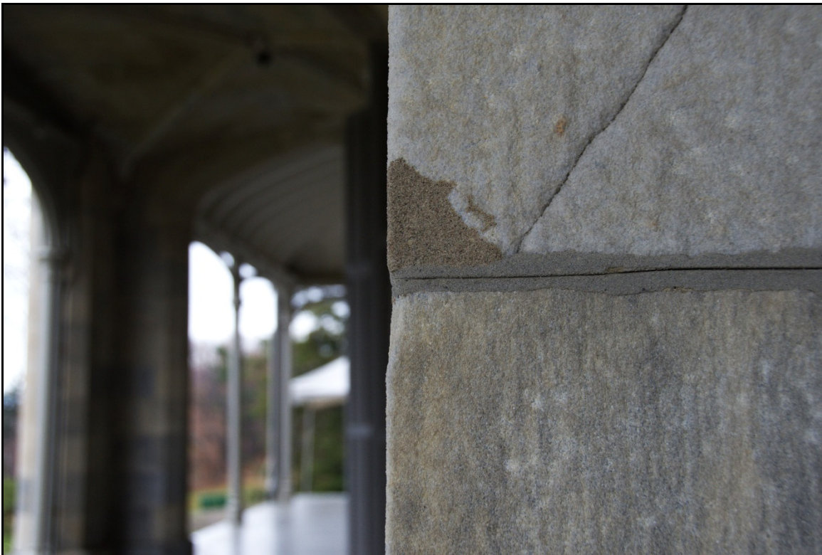
Figure 4. 5: Detail of portland cement and resulting material loss and cracking (Photo by author).
