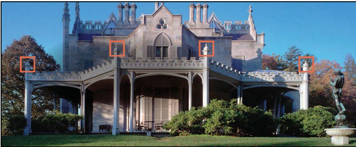
Figure 4.22: Location of mansion roof finials on south elevation (Photograph courtesy of Lyndhurst website and altered by author).
