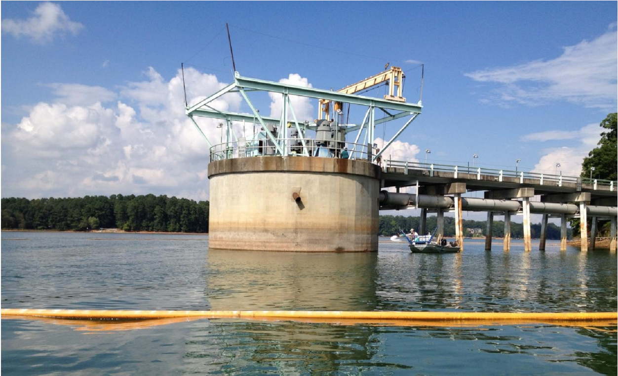
FIGURE 2. Anderson Regional Joint Water System intake structure on Hartwell Lake.
