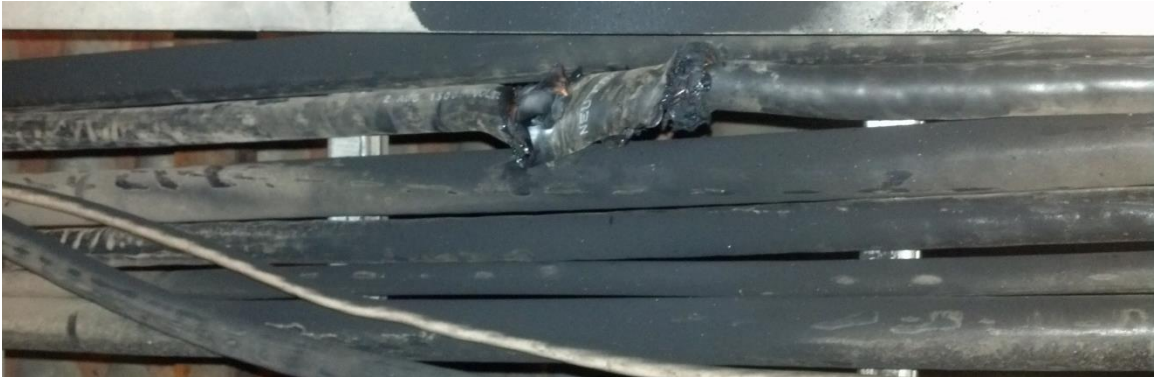
Figure 1.1: Short circuit in underground cable in conduit in Clemson
