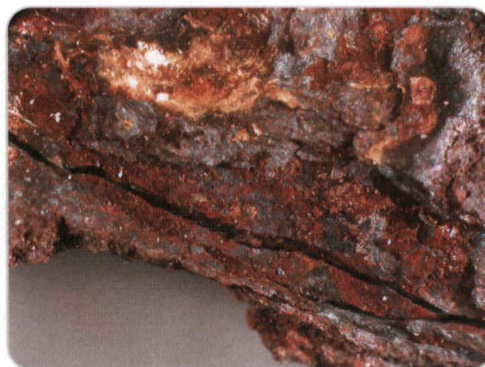
Microscopic View: cracking
