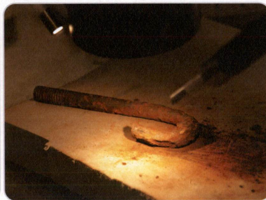
Photograph 11: Post mechanical treatment view of threaded hook
