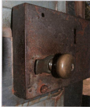
Photograph 2: View of lock in place
