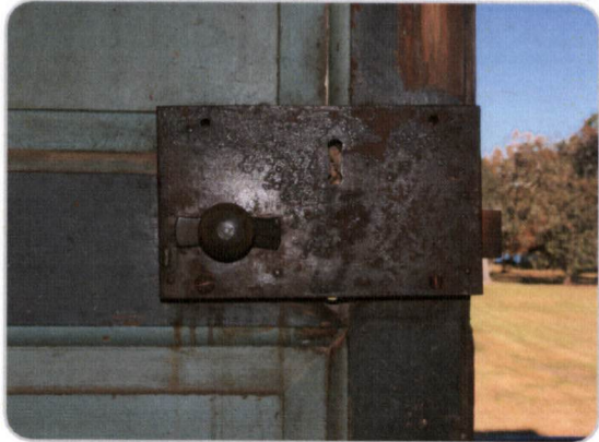
Photograph 1: View of lock in place
