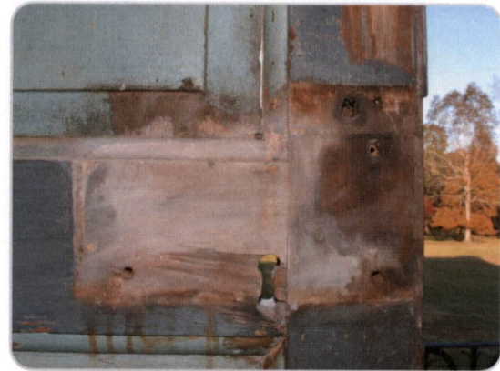
Photograph 3: View of door without lock, note multiple bolt and keyholes
