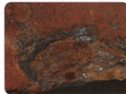
Post Treatment View: close up pitting
