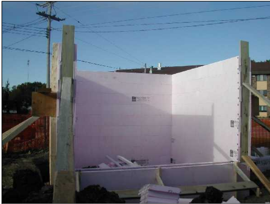
Figure 5.13: Laura Ingalls Wilder Museum Dugout Replica building form (Laura Ingalls Wilder Museum)
