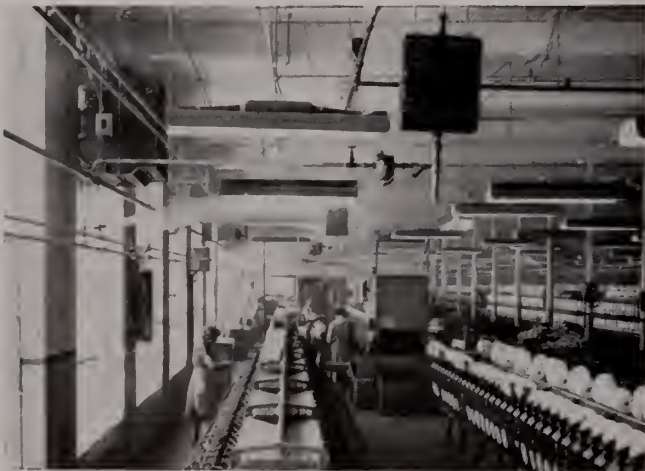
AMCO Evaporative Cooling System in Texas Textile Mills, McKinney, Texas. Note window units which control mixture of fresh and recirculated air.
