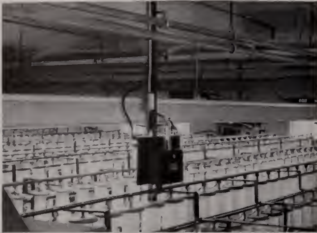
AMCO Humidification System installed at Caron Spinning Company, Rabesonia, Pa. The highly sensitive AMCO Cyclestat Control holds humidity within narrow limits
