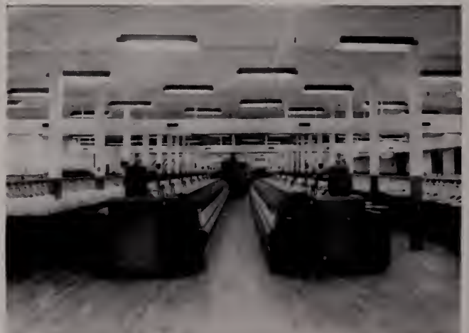
AMCO Central Station Air Conditioning in the Raving Dept., Highland Park Mills, Charlotte, N. C. This is AMCO's highly efficient split-system.
