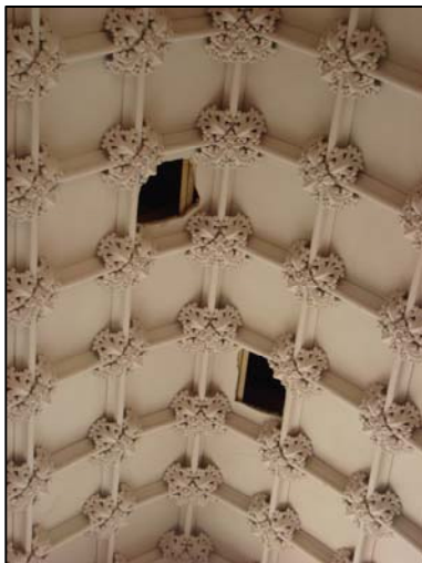
Figure 122. Holes cut in the Chancel ceiling to inspect and monitor termite damage. (Photo: Author)
