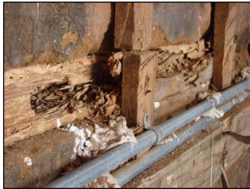
Figure 114. Termite trails on original support beams in the pisé wall. (Photo: Author)
