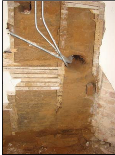
Figure 137. View of eastern pisé wall from inside the Sacristy. The hole that the metal pipes are going through goes all the way through the wall. (Photo: Author)
