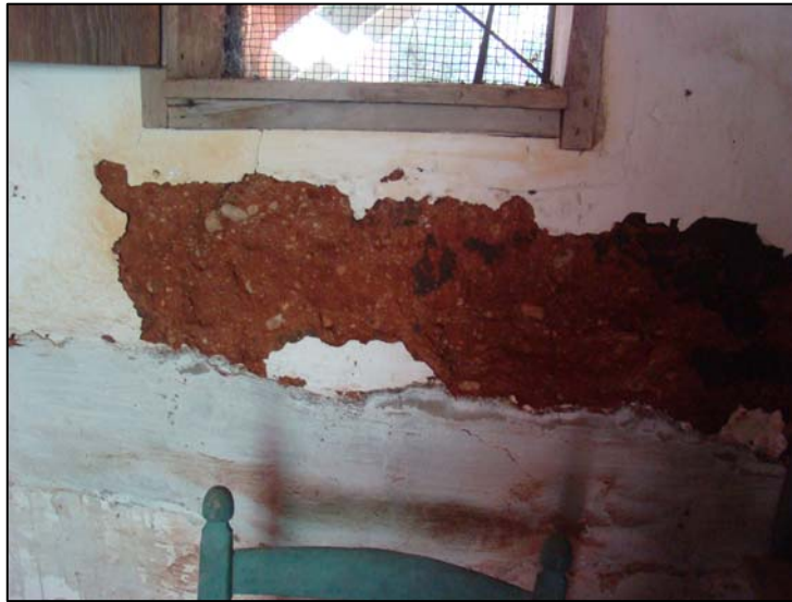
Figure 98. Interior wall showing some plaster loss inside the dairy/kitchen. (Photo: Author)
