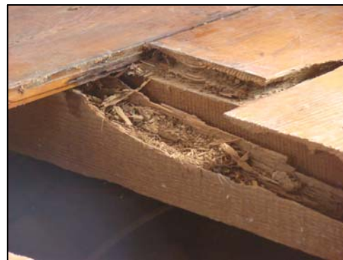
Figure 117. Severe termite damage on floorboards under choir area. (Photo: Author)
