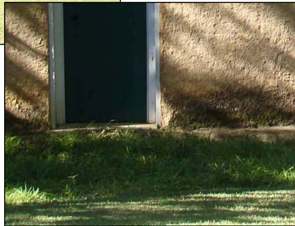
Figure 93. Closer view of the staining. (Photo: Author)
