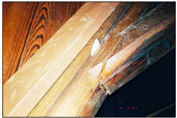
Figure 128. The arrow points to the area where the roof truss has pulled away from other wooden members because of weakened structure. (Photo: Cummings and McCrady Architects)
