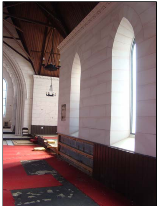
Plate A22. Concrete block repair made after the collapse of a portion of the south wall in 1974. (Photo: Author)
