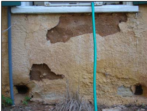
Figure 83. Loss of pebble dash on the eastern wall of the doctor's office due to water leaking from the air conditioning unit. (Photo: Author)
