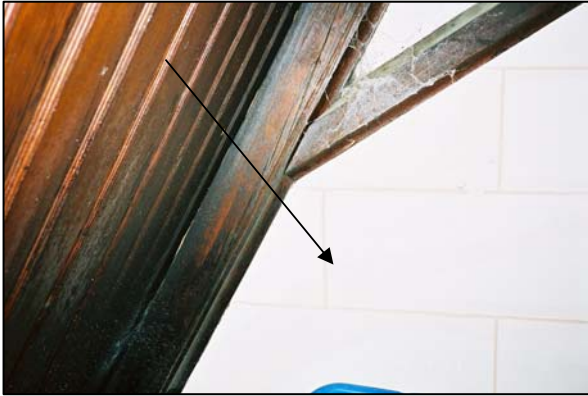
Figure 125. Arrow points to cracking in roof truss due to termite damage and weakened strength. (Photo: Cummings and McCrady Architects)
