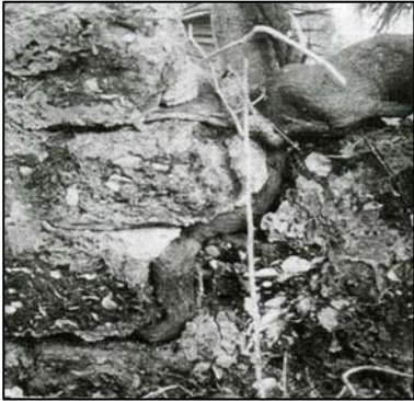
Figure 13. Vine damage in a tabby wall. (Photo: Lauren B. Sickels – Taves.)
