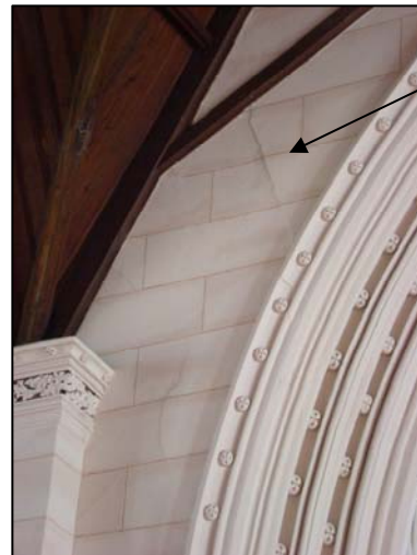
Figure 123. Arrows point to cracks due to weakened structure. (Photo: Author)
