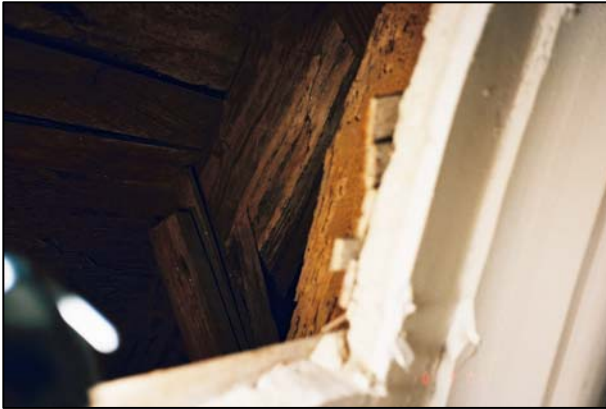
Figure 129. This is a view through a hole cut in the Chancel ceiling showing extensive termite damage in the roof structure. (Photo: Cummings and McCrady Architects)
