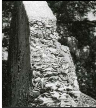
Figure 14. Damaged tabby wall with previous cement repairs at top. (Photo: Lauren B. Sickels- Taves)
