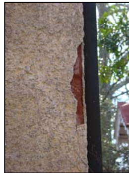
Figure 100. Closer view of area of pebble dash loss (about six inches in length) (Photo: Author)
