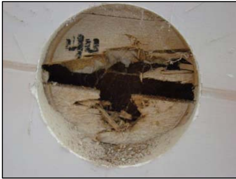
Figure 118. Holes cut in plaster to monitor termite damage. (Photo: Author)
