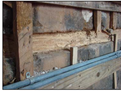
Figure 115. Termite trails on original support beams in the pisé wall. (Photo: Author)
