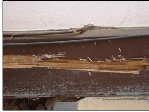
Figure 113. Termite trails on the baseboard in the Chancel. (Photo: Author)
