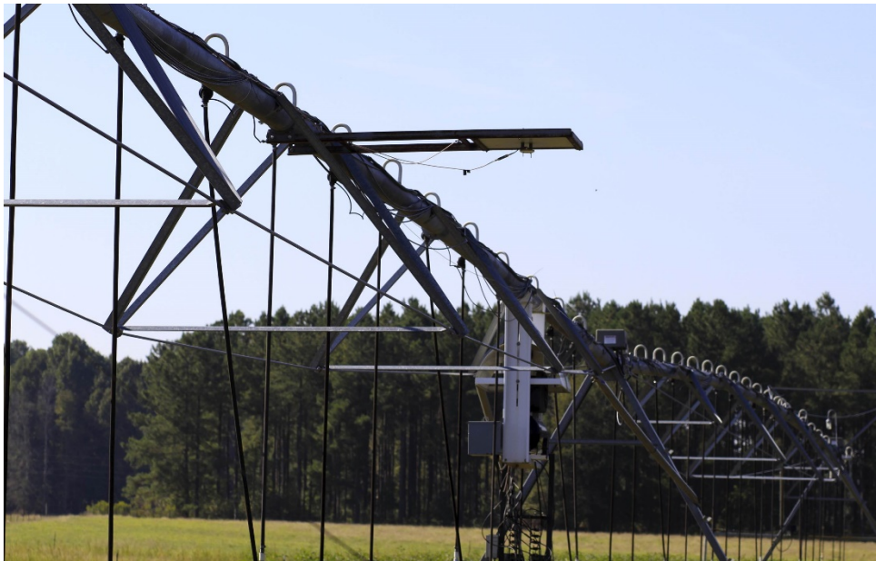
Figure 2.6 GPS antennas mounted on VRI during 2013 growing season
