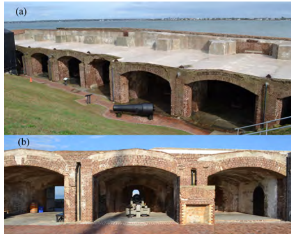
Figure 54: System of casemates at Fort Sumter showing (a) the Right face and (b) the Left flank of the fort.
