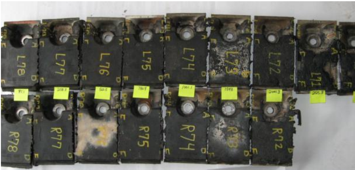
Figure 1.3. Track Backer Pad Failures Due to Chunking [2]
