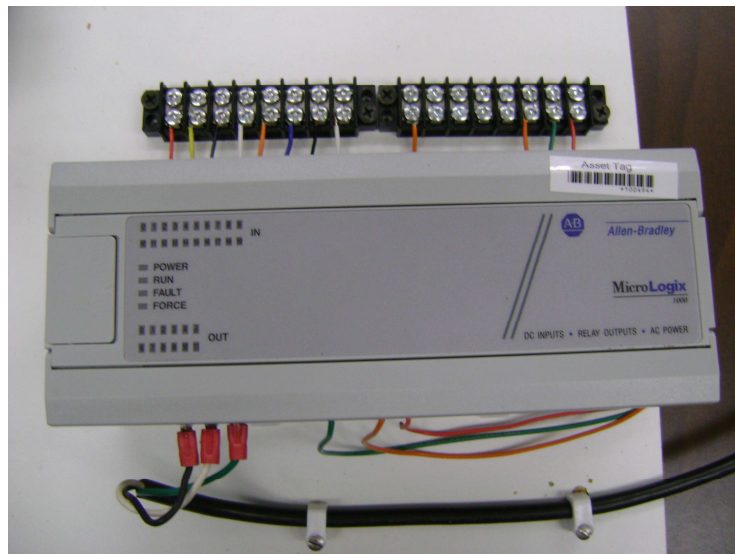
Figure C-1: Allen Bradley MicroLogix 1000 PLC [23]
