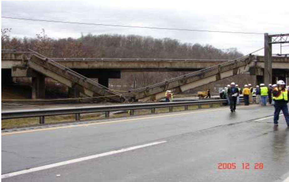
Figure 2.15: Lakeview Drive Collapse (Scott 2006)
