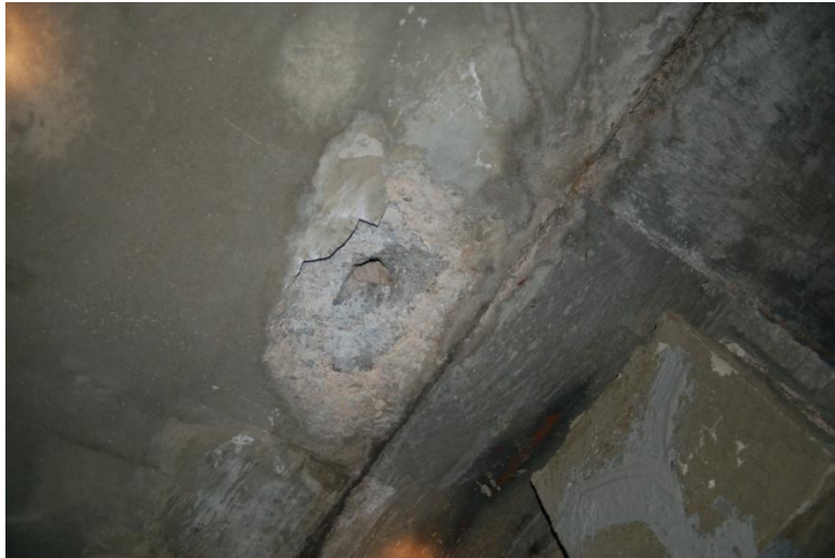
Figure C-7. James B. Edwards Bridge: Large Spall in Segment Roof near Joint
