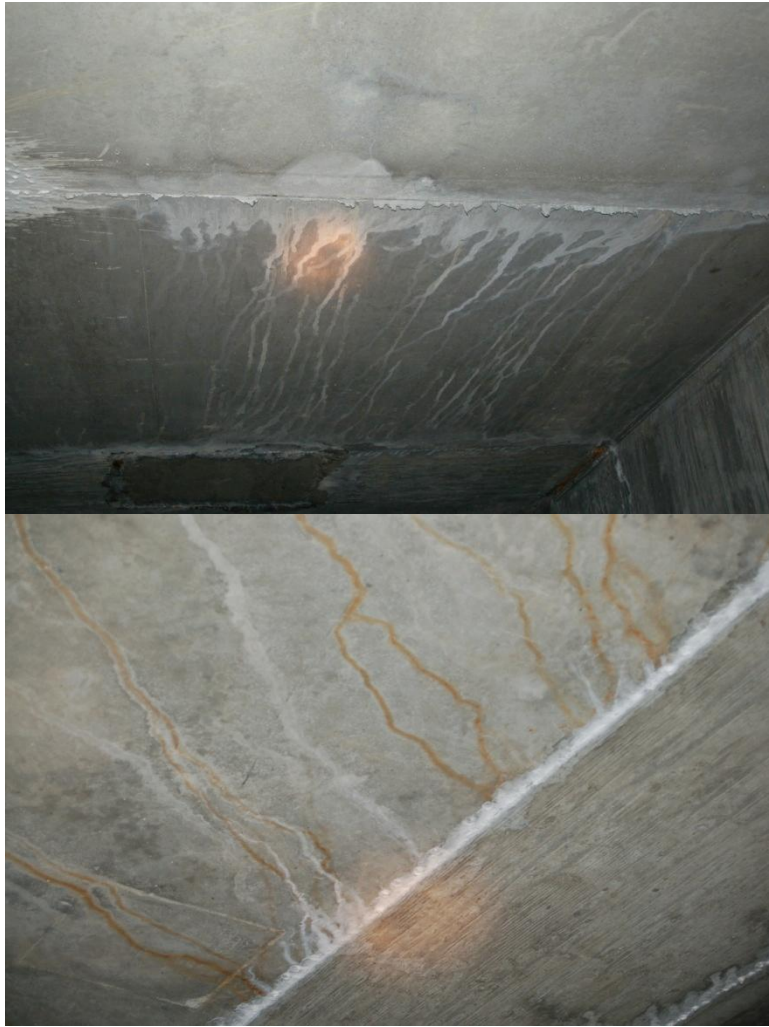
Figure C-5. James B. Edwards Bridge: Efflorescence from Leaky Joints
