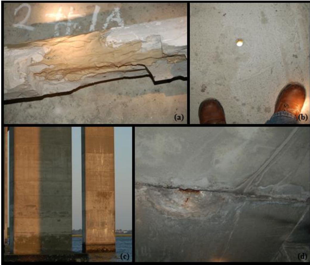
Figure 3-5. SCDOT Inspection of James B. Edwards Bridge: (a) Improper Grouting of Ducts (b) Small Void Drain Holes (c) Cracks in Piers (d) Leaky Joints
