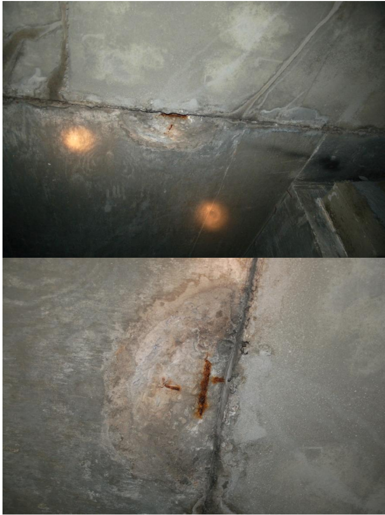
Figure C-6. James B. Edwards Bridge: Leaky Joint with Exposed Rebar
