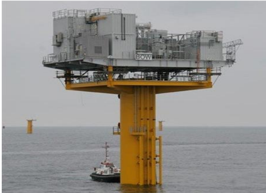
Figure 4.2 Picture of offshore substations [10]
