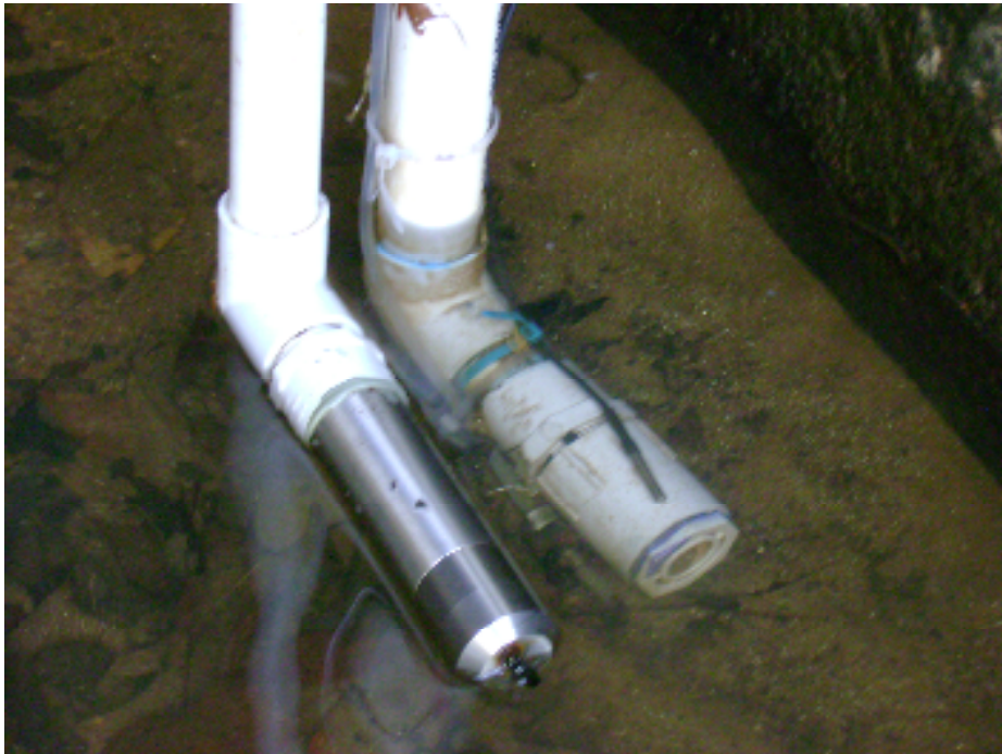
Figure 28. Turbidity sensor, bubbler, temperature sensor, and pressure transducer installed in Honeycutt Creek.
