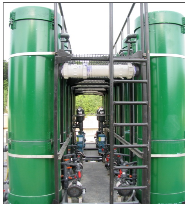
Figure 12: Ammonia Recovery Process at "landfill site II", showing green de-sorption columns and leachate recycle pumps.
