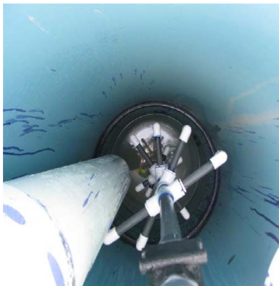
Figure 9: Internal view of absorption column showing spray nozzles.
