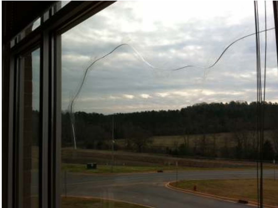
Figure 4.7. Photograph of cracking windows by Principal Portsmouth.
