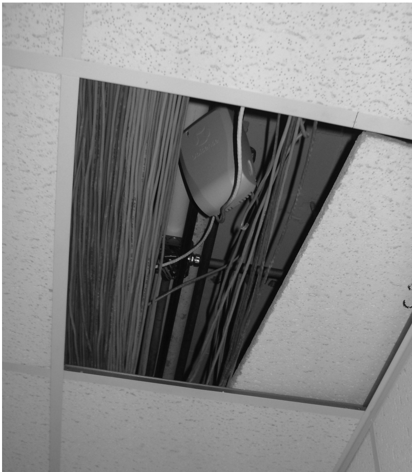
Figure 2.10: Photo of a sensor installed in the Riggs facility.
