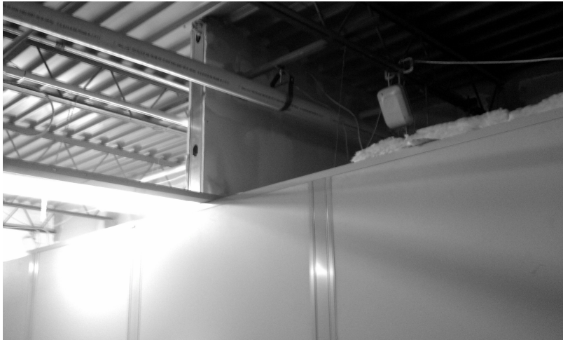
Figure 2.9: Photo of a sensor installed in the Shoothouse facility.
