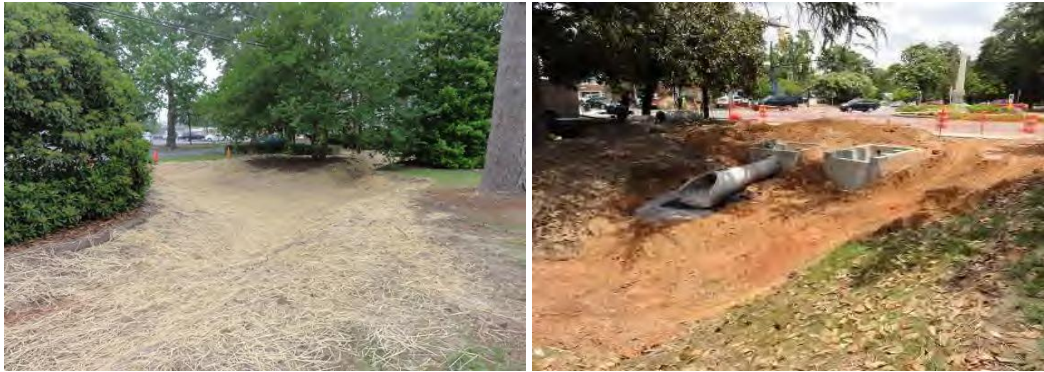
Figure 4-1. The bioretention cell between Richland Avenue and Park Avenue along Chesterfield Street (CRP) during construction.
