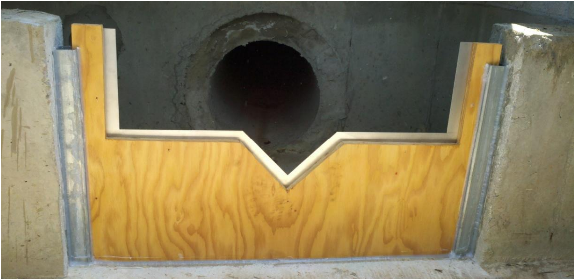
Figure 4-5. Post-installation picture of combination weir configuration at the inlet of the bioretention cell between Newberry and Laurens Streets along Park Avenue (Bellamy, 2010).
