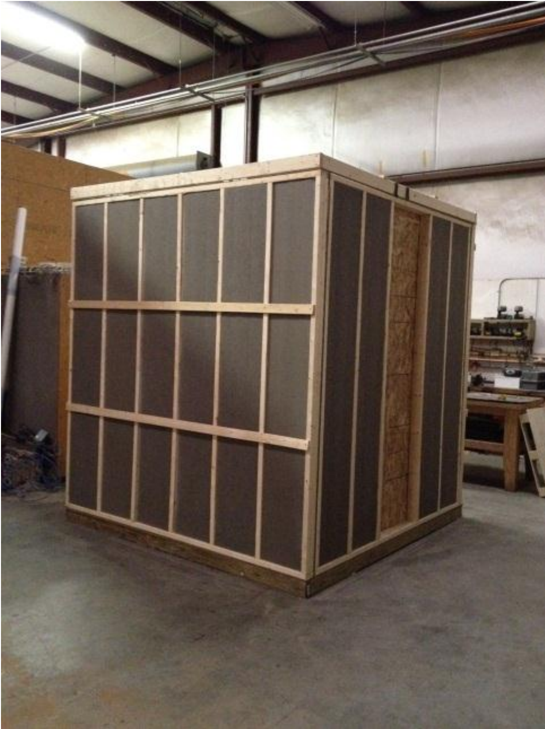
Figure 3-6: The unfinished experimental room with the insulation missing between the two studs where the two inlet location were installed
