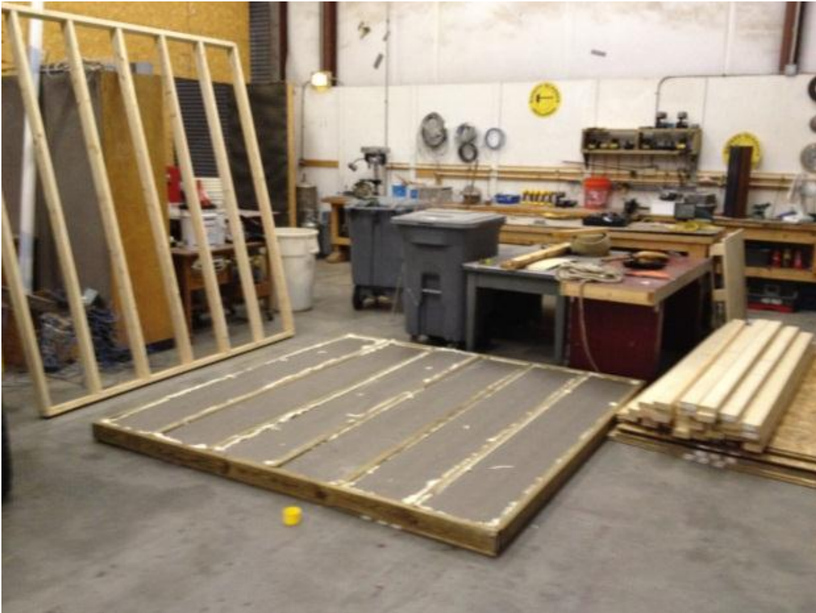
Figure 3-1: The Base wall insulated on the floor and one framed wall braced, standing up
