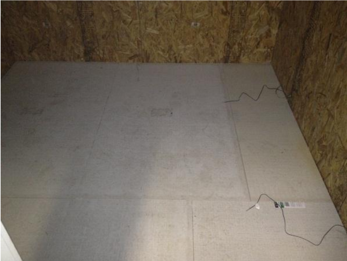
Figure 3-8: The thermocouples that are attached to the thermostats for the under floor distributed heating system
