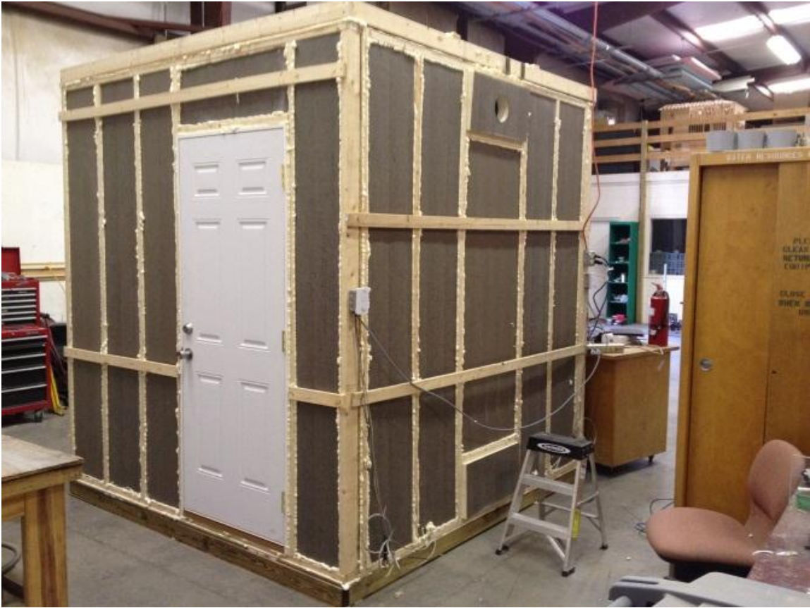
Figure 3-5: The final experimental room
