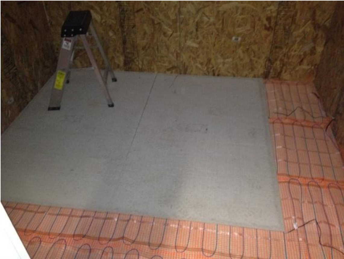
Figure 3-7: The under floor distributed heating system partially covered in cement board
