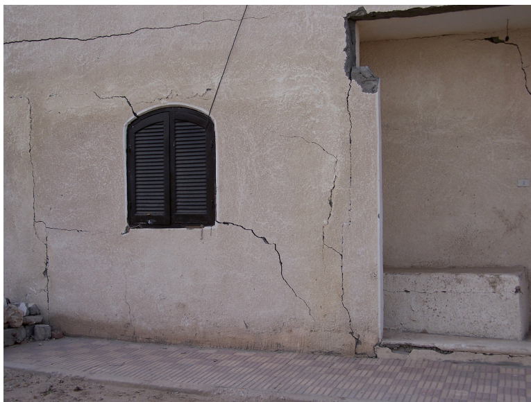
Photo 6.2. Homes with Structural Problems (by Author).
