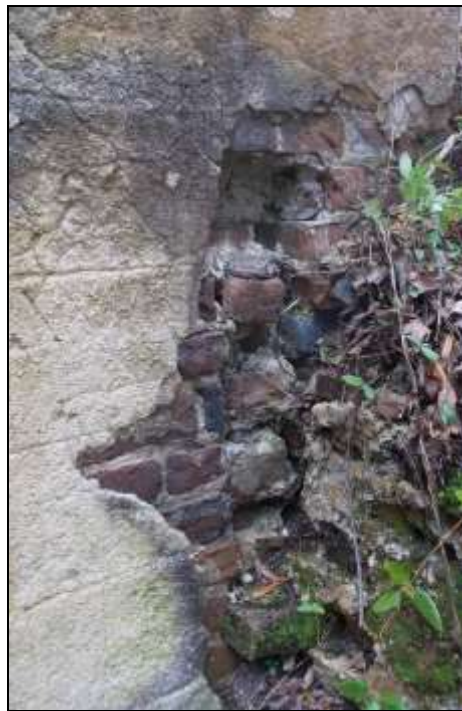
Figure 24. Landside elevation, west side of the portico, showing pockets for decorative cladding.
