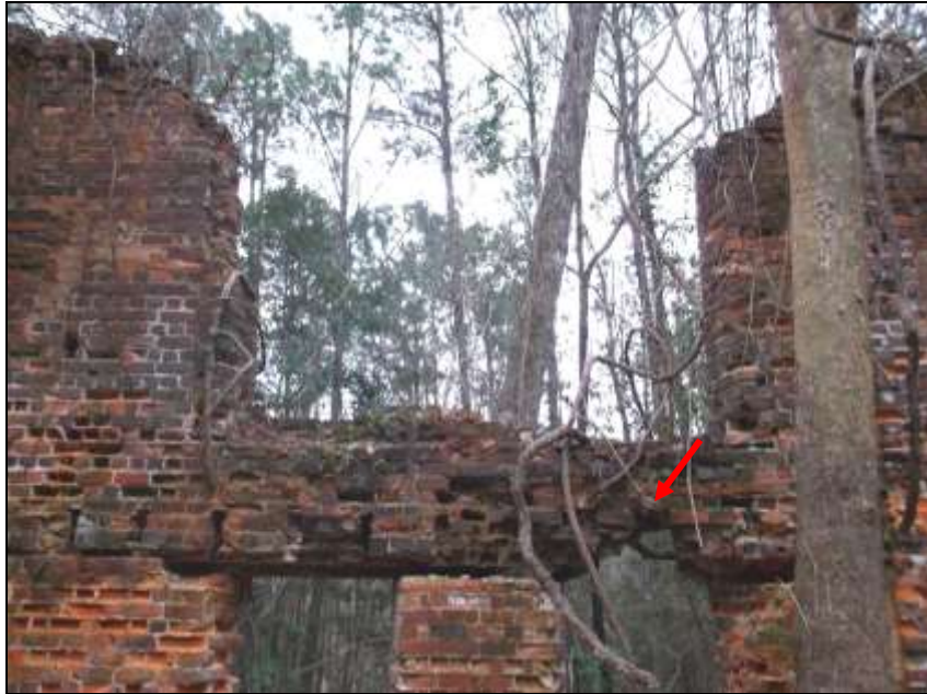
Figure 107. East elevation interior, central bays, showing missing wall between bays 3 and 4 and missing bricks in bay 3.
