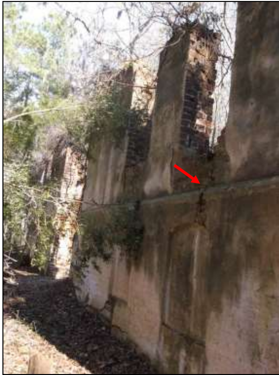
Figure 116. West elevation, southern extent showing crack in bay 5.
