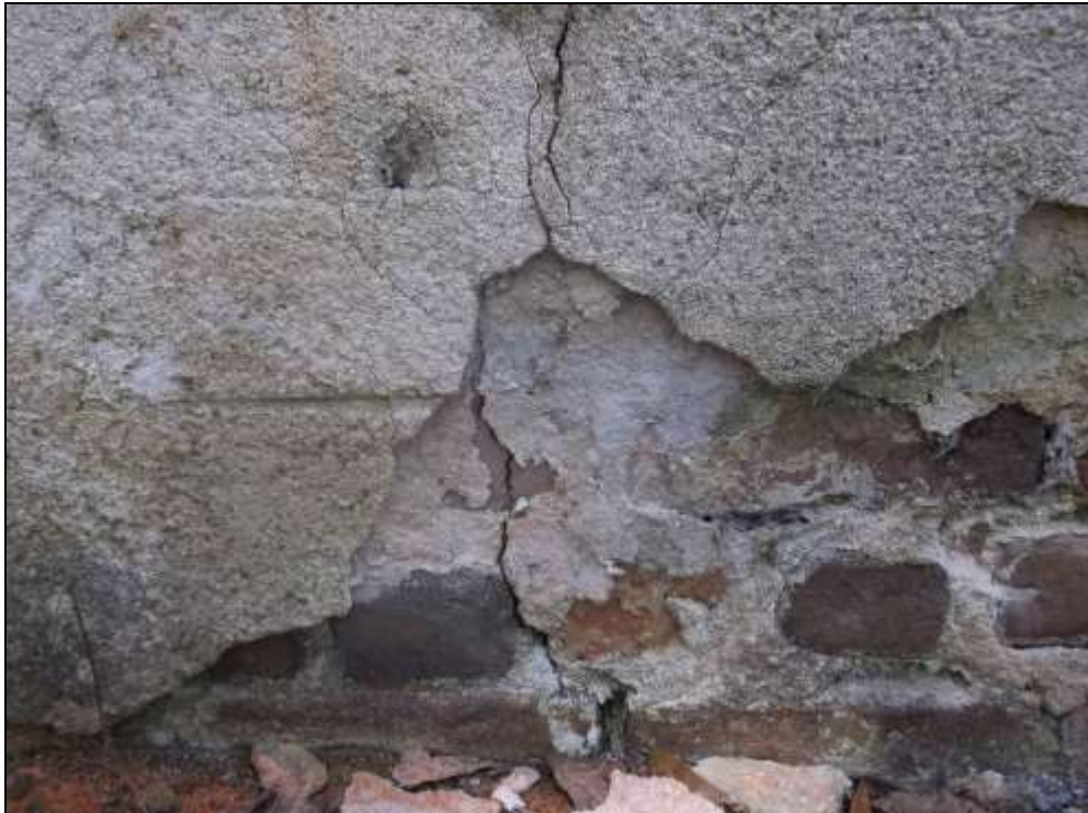
Figure 112. East elevation, northern extent, close-up of foundation crack.
