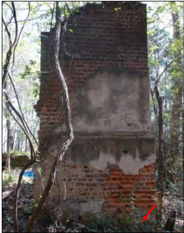
Figure 101. Location of foundation crack in landside elevation eastern extent.
