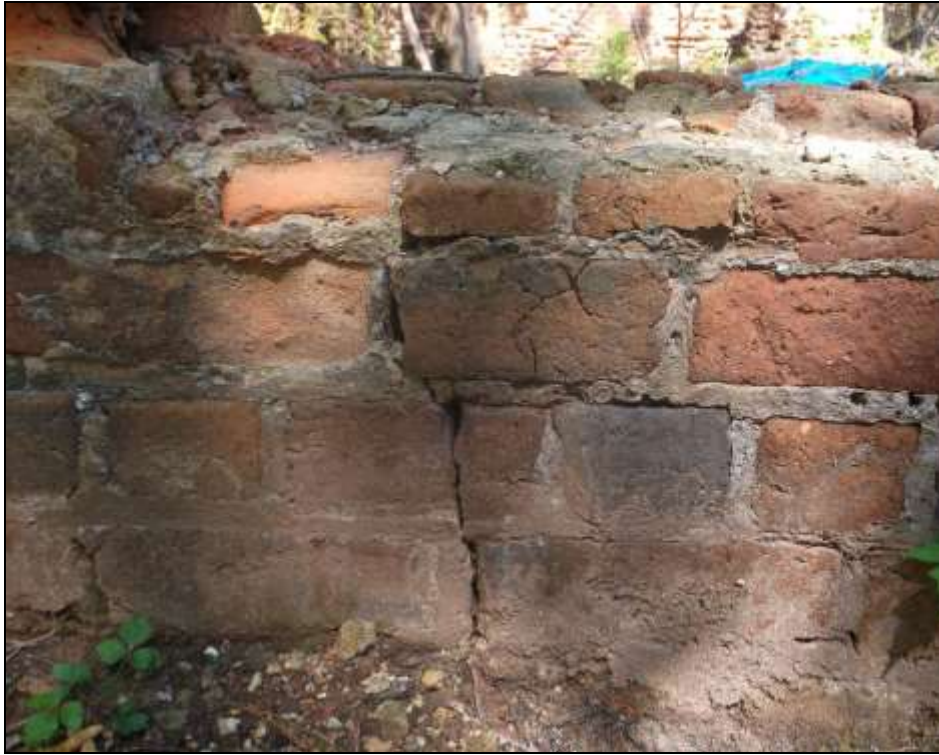
Figure 105. East elevation, bay 2, showing cracking below the window opening.
