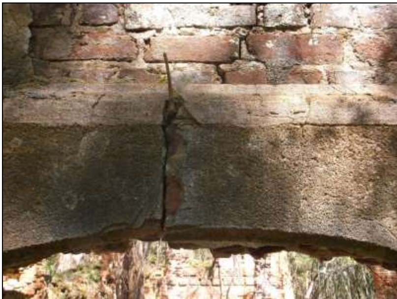
Figure 104. East elevation, bay 2, showing cracking above the window opening.
