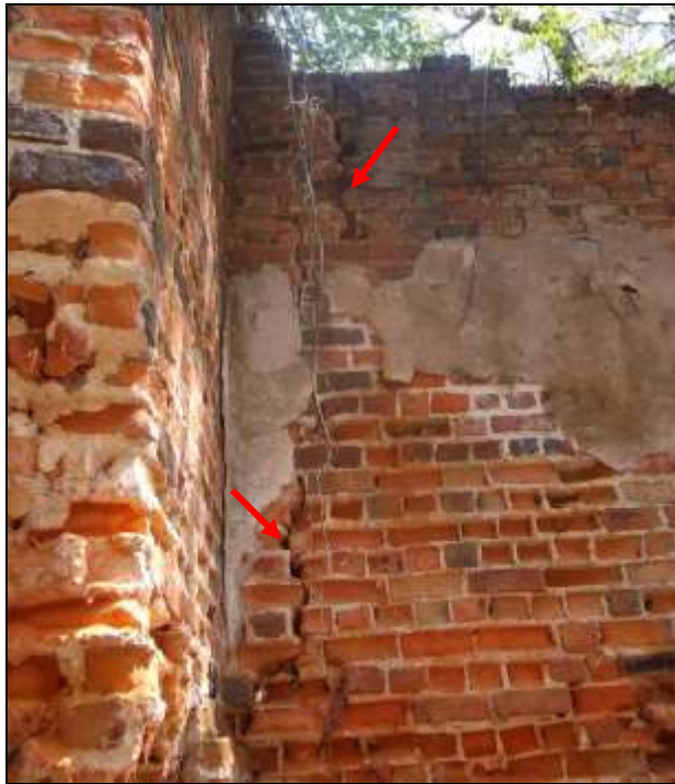
Figure 113. East elevation interior, northern extent, showing structural cracking at the northeast corner.
