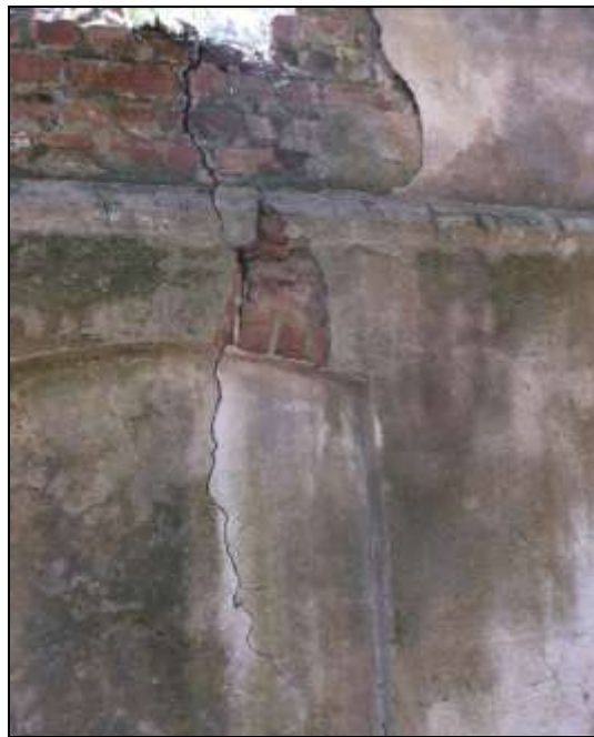
Figure 117. Close-up of crack in upper window sill through to blind window in bay 5, western elevation.
