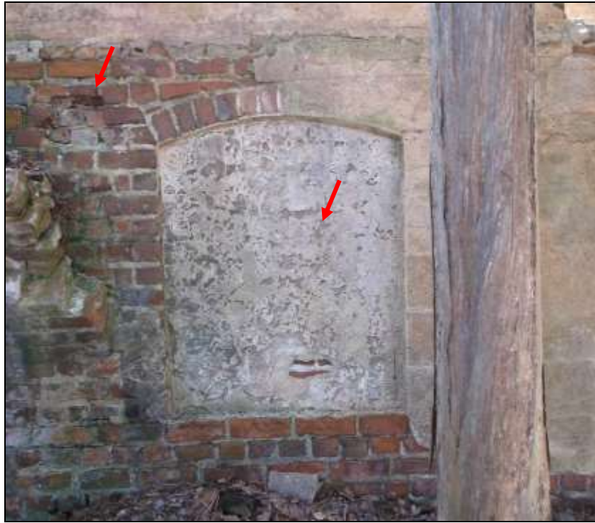
Figure 34. The remnants of decorative elements, riverside portico.
