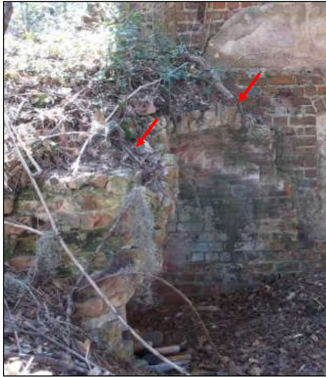
Figure 97. Western extent of the riverside portico showing damage by vegetation.
