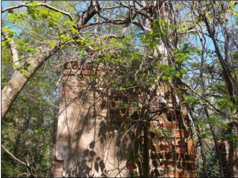
Figure 99. Interior wall remnants showing vegetation growth at the top of the wall.
