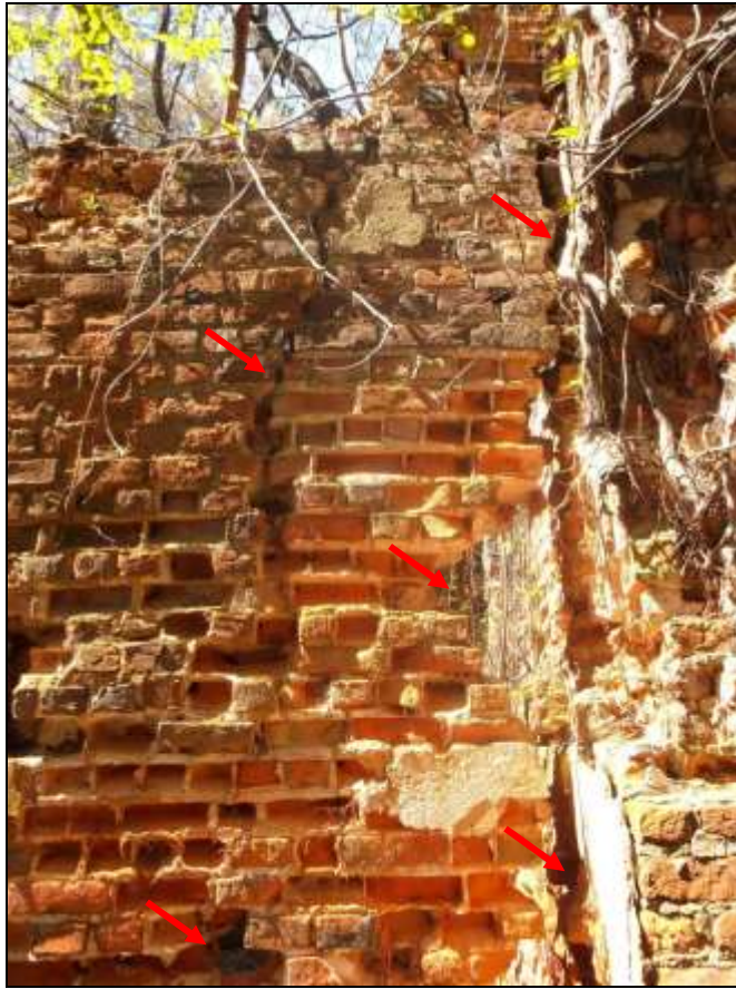
Figure 119. West elevation, southern interior wall, showing erosion and broken tie-in; view southwest.
