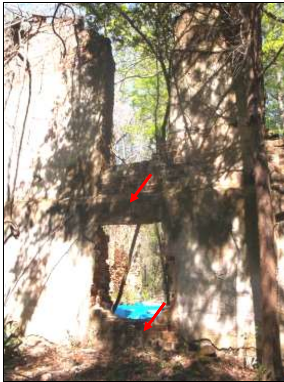
Figure 108. East elevation, bay 5 overview. Showing location of cracked window sills.
