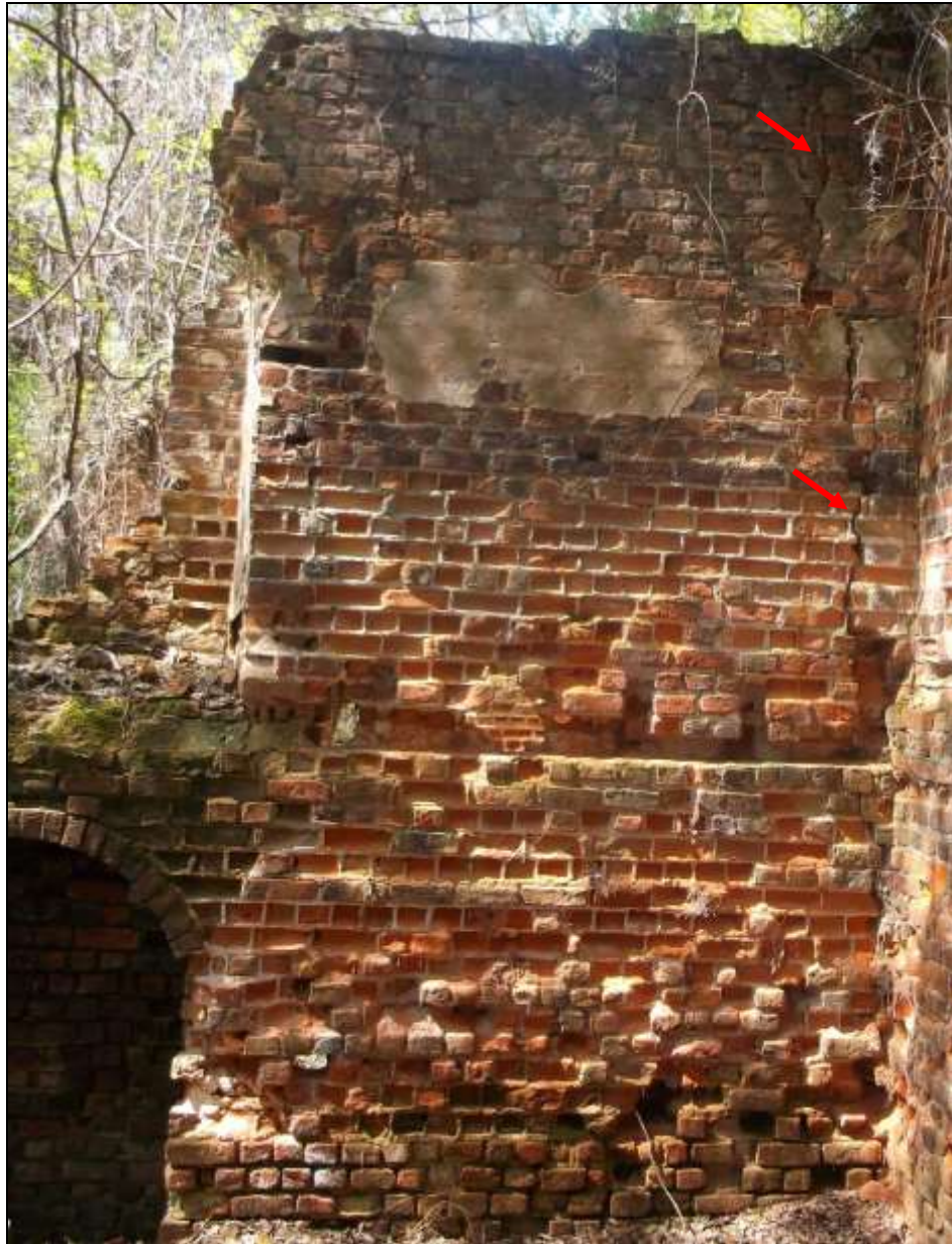
Figure 120. West elevation, northern interior wall showing structural cracking near the tie-in and eroded brick and mortar.
