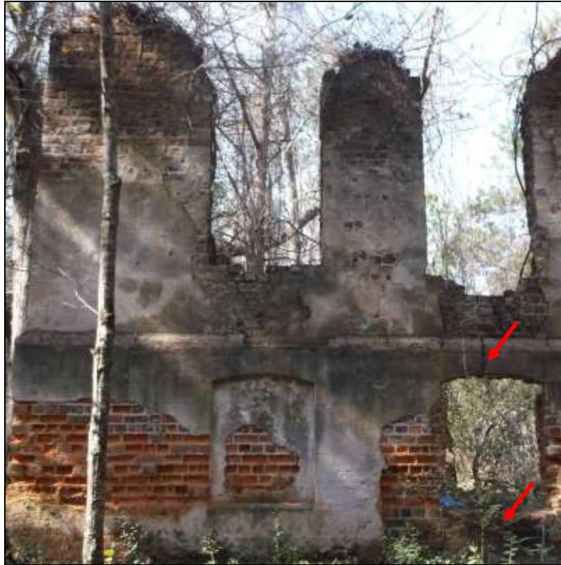
Figure 103. East elevation, southern extent showing bays 1 and 2, and crack in window sill in bay 2.
