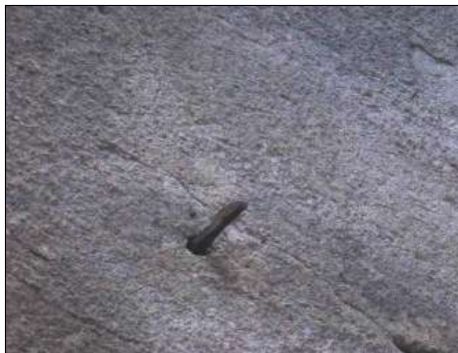
Figure 25. Photo showing the remnants of an iron shutter dog next to a window on the west elevation.
