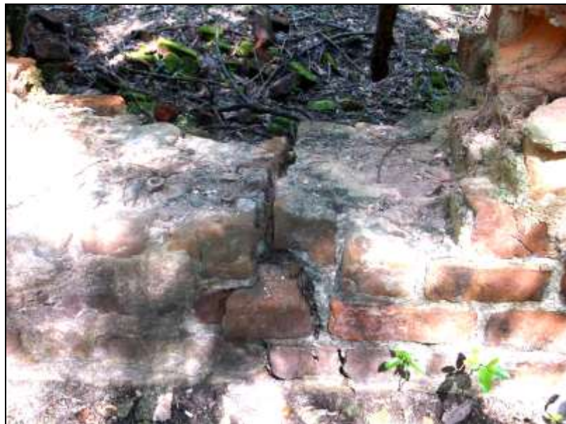
Figure 110. East elevation bay 5, close-up of crack through bottom window opening.
