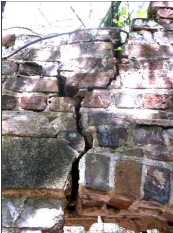
Figure 109. East elevation bay 5, close-up of crack between upper and lower window openings.
