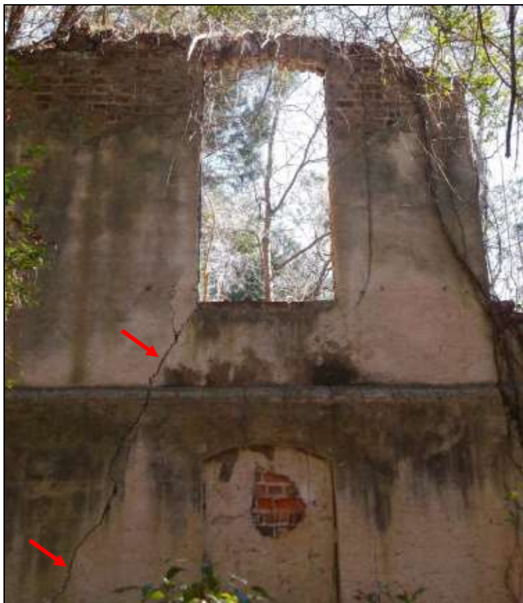
Figure 115. West elevation, northern extent, showing structural crack at the window opening.
