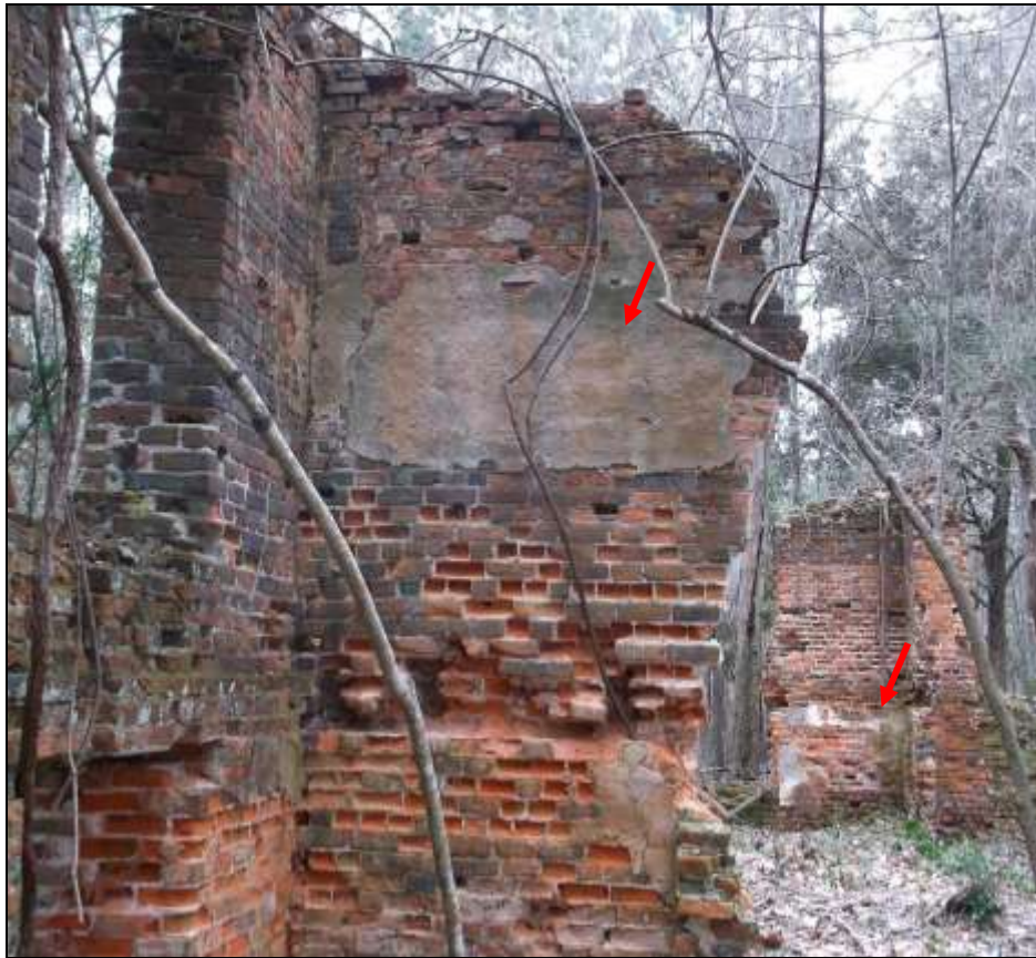
Figure 51. Interior eastern elevation showing the remnants of plaster on interior walls.
