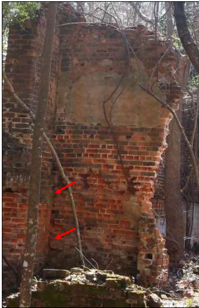
Figure 118. East elevation interior T-wall remnant, showing structural cracking near intersection of walls.
