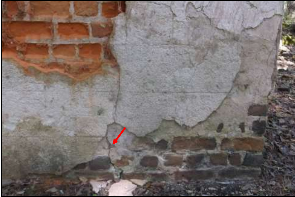
Figure 111. East elevation, northern extent, showing foundation crack.
