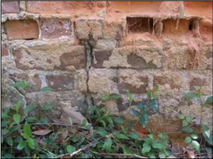
Figure 102. Close-up of foundation crack, landside elevation, eastern extent.
