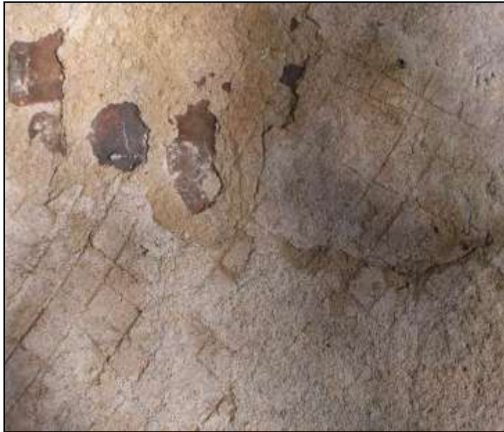
Figure 21. Stucco remnants showing scratch coat.
