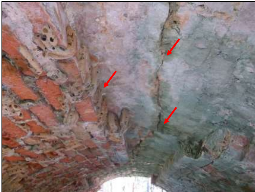
Figure 98. Interior of the riverside portico tunnel arch showing water damage, missing brick and structural crack.
