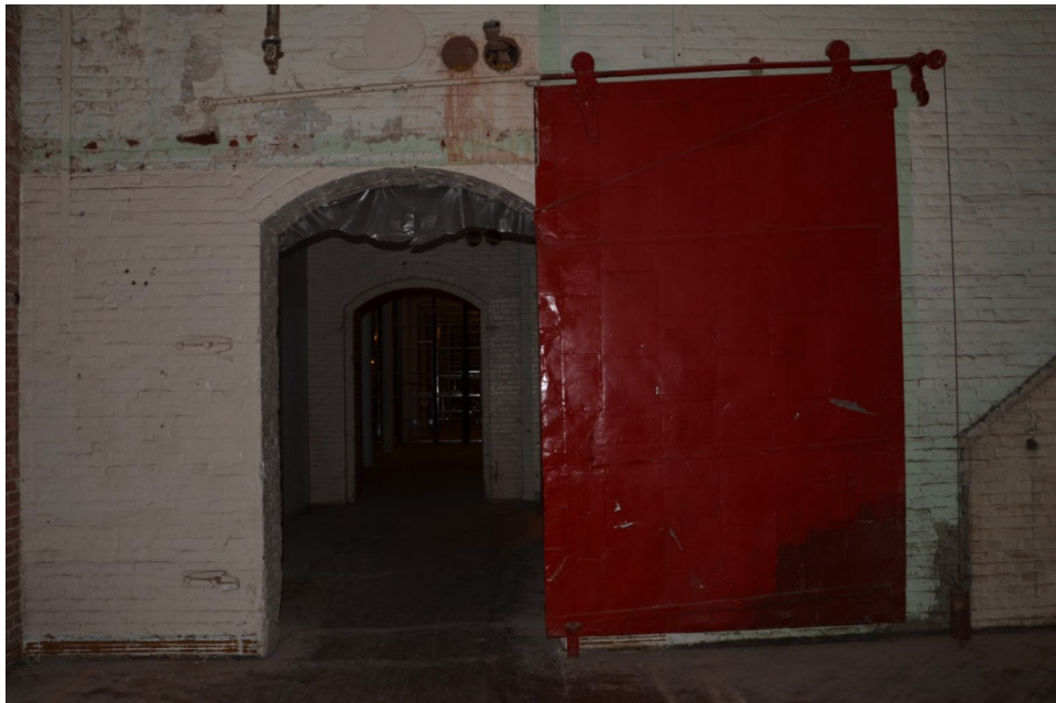
Figure 3-12. Image showing a sliding fire door system with attached rope pulley at the Cigar Factory, Charleston, South Carolina. Photo by author.
