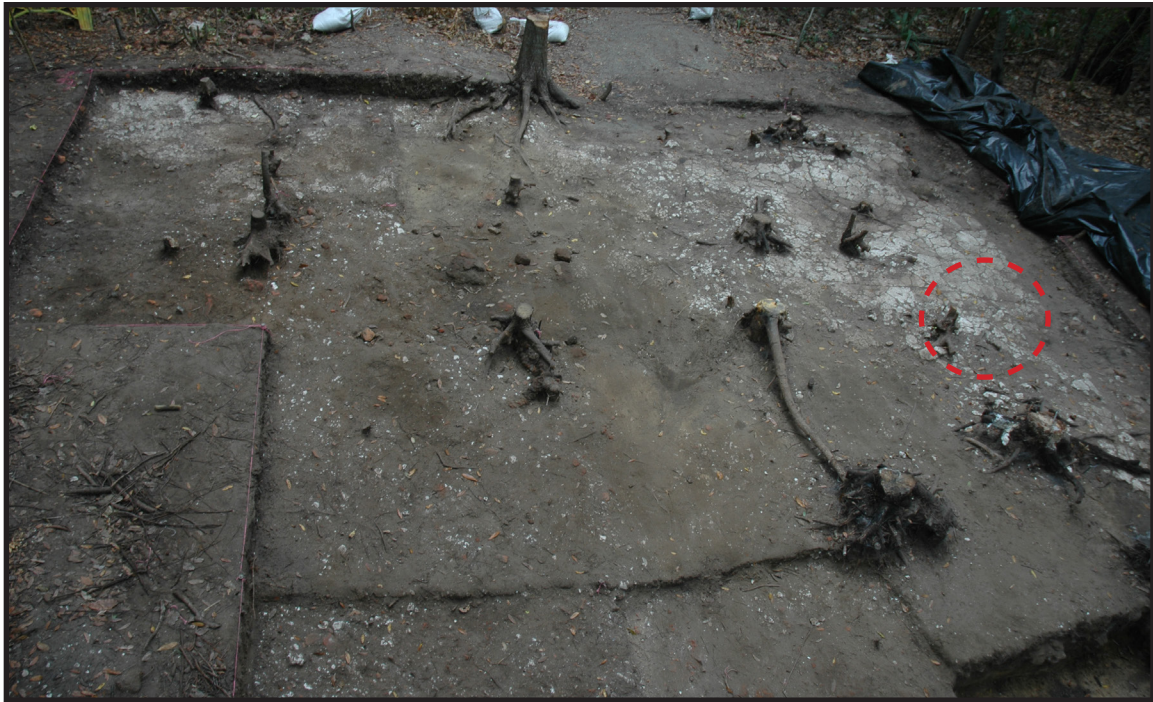
Figure 13. Image showing Extents of Miller Site Tabby Floor and Approximate Location Sampling Identified (Photograph by Charles Towne Landing, 2010).
