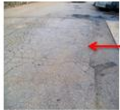
Irregular ground surface
