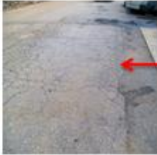
Irregular ground surface
