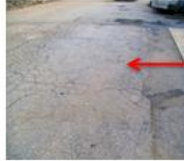
Irregular ground surface
