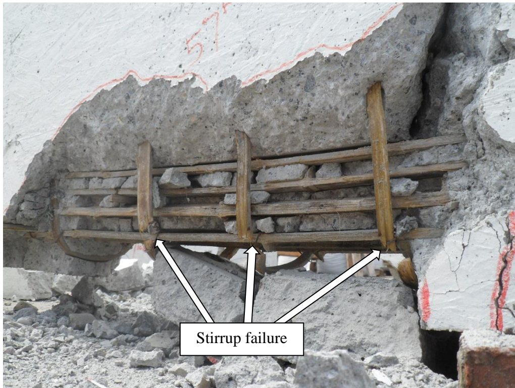
Figure 7.34 Stirrup failure in front face of beam L3
