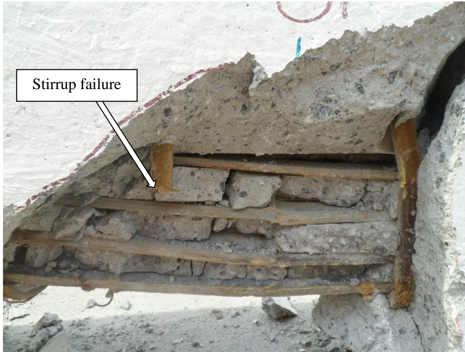
Figure 7.32 Stirrup failure in front face of beam L2
