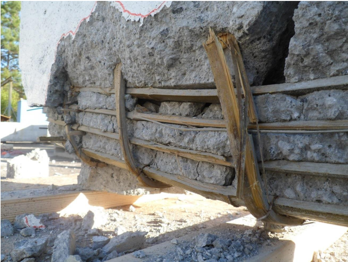
Figure 7.8 Failure in middle of bamboo stirrup of beam S3
