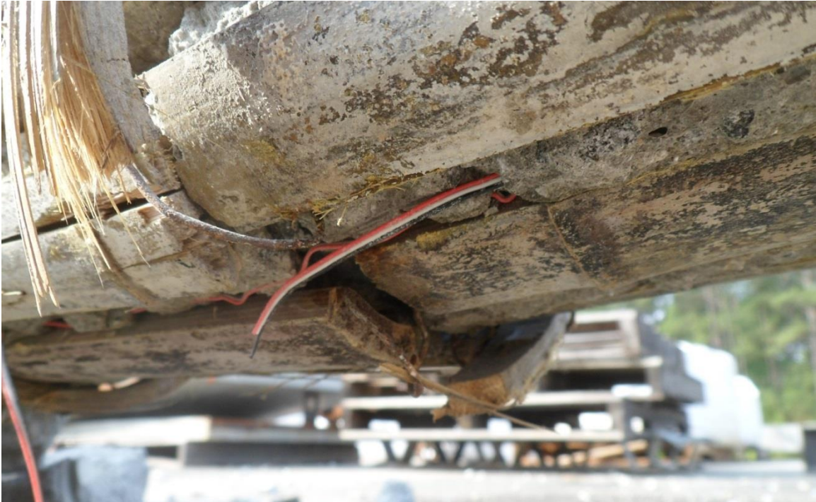
Figure 7.22 Longitudinal failure at stirrup location in beam F4
