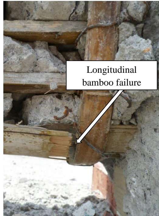
Figure 7.21 Longitudinal bamboo failure in beam F1 (close-up)
