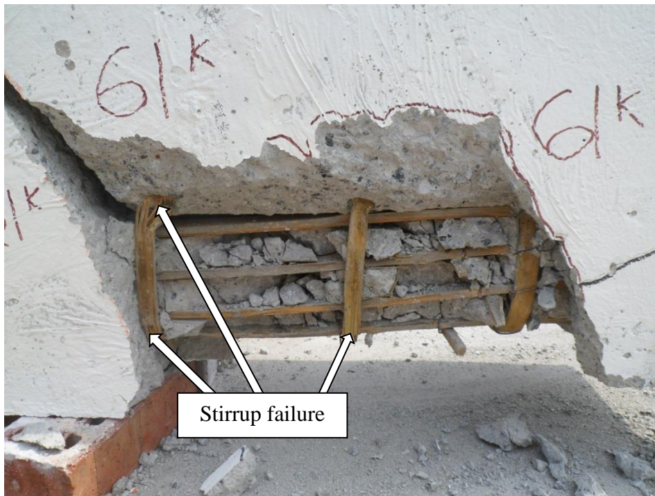
Figure 7.33 Stirrup failure in back face of beam L2
