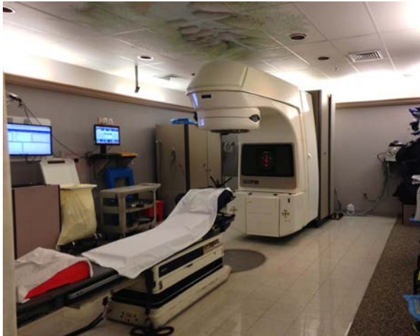
Figure 62: an older vault at the Lancaster Cancer Centre, with institutional clutter around LinAc (Braden Reid)
