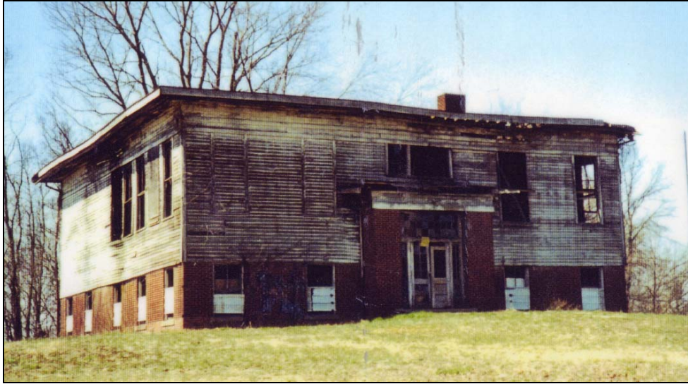
Figure 1: Lyles Consolidated School before reconstruction. Photograph from the Lyles Station Historic Preservation Corporation.
