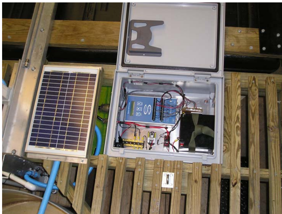
Figure 3.17: Data Logger and Electronic Setup
