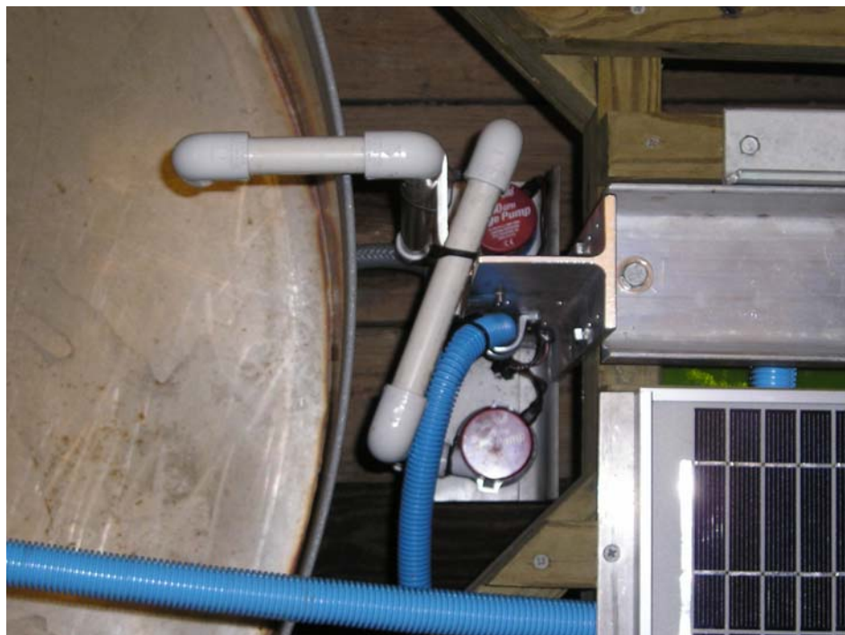
Figure 3.13: Pump System (top view)
