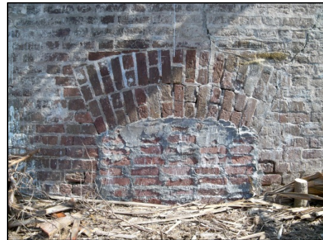
Figure 7.6 Bricked up opening
