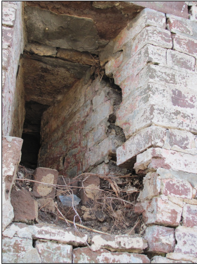
Figure 7.19 Showing large stress fracture in opening
