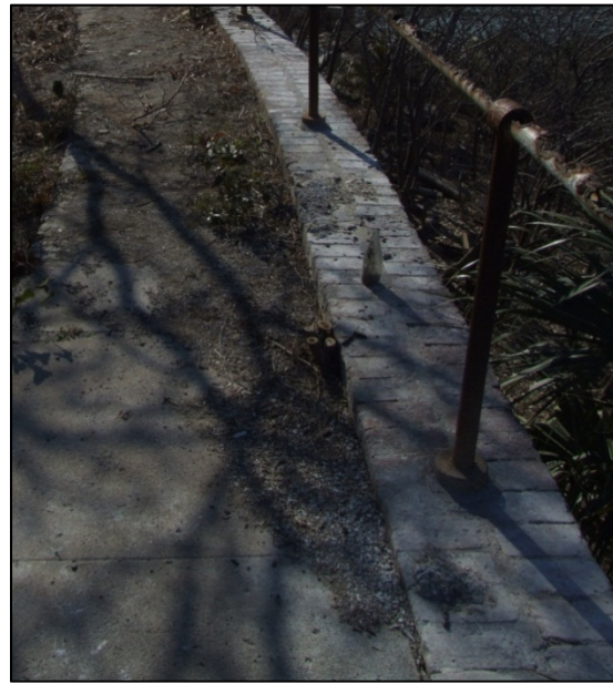
Figure 7.9 Large tree growth on top of wall
