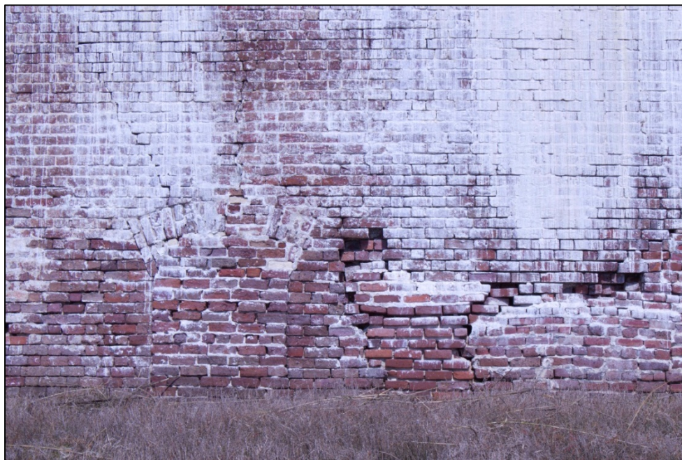
Figure 7.14 Showing diagonal fracturing above embrasure arch and adjacent under fired brick erosion
