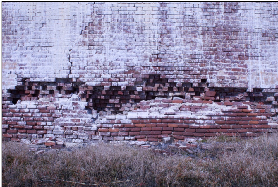
Figure 7.15 Showing erosion caused by water at base of the wall, and resultant brick loss and stress fracturing
