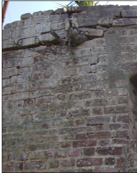
Figure 7.21 Showing large plant growth and resultant fracturing
