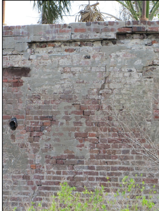
Figure 7.5 Further damage caused by Portland cement; brick and mortar loss
