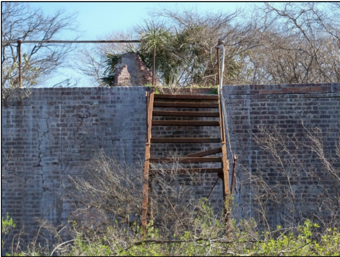
Figure 7.7 Showing both stress fracturing and fracturing due To incompatible masonry
