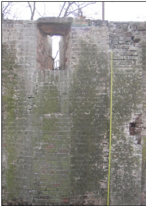
Figure 7.23 Showing exposed brownstone header and brick displacement
