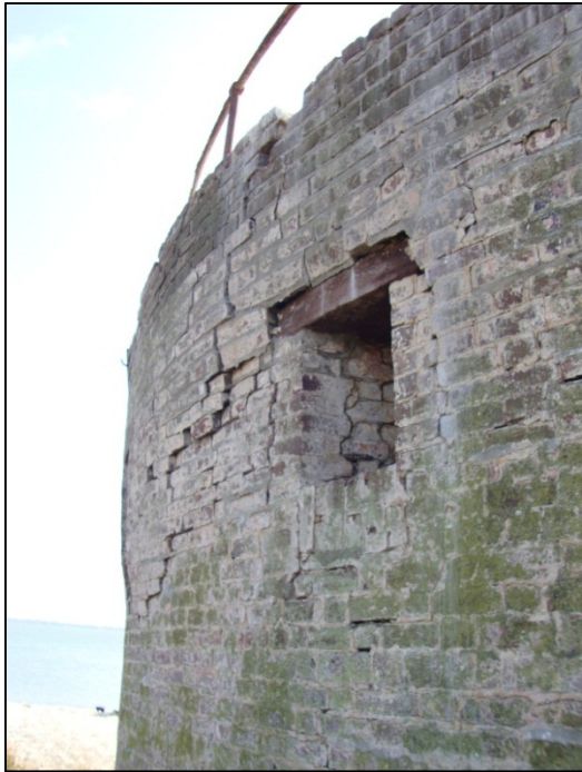
Figure 7.20 Showing wall leaning and fracturing due to settlement
