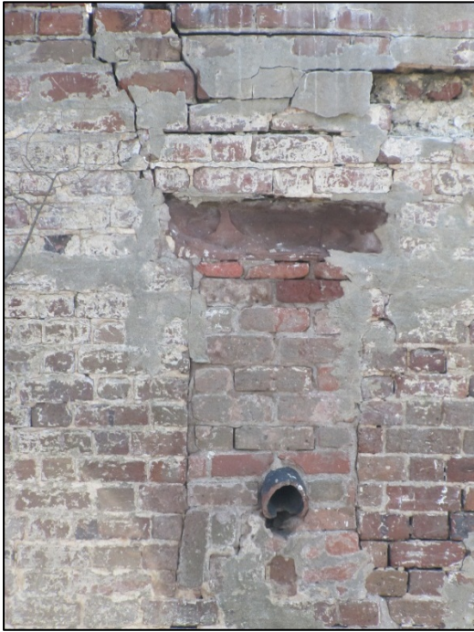
Figure 7.4 Damage caused by Portland cement; spalling brownstone header and fracturing brick
