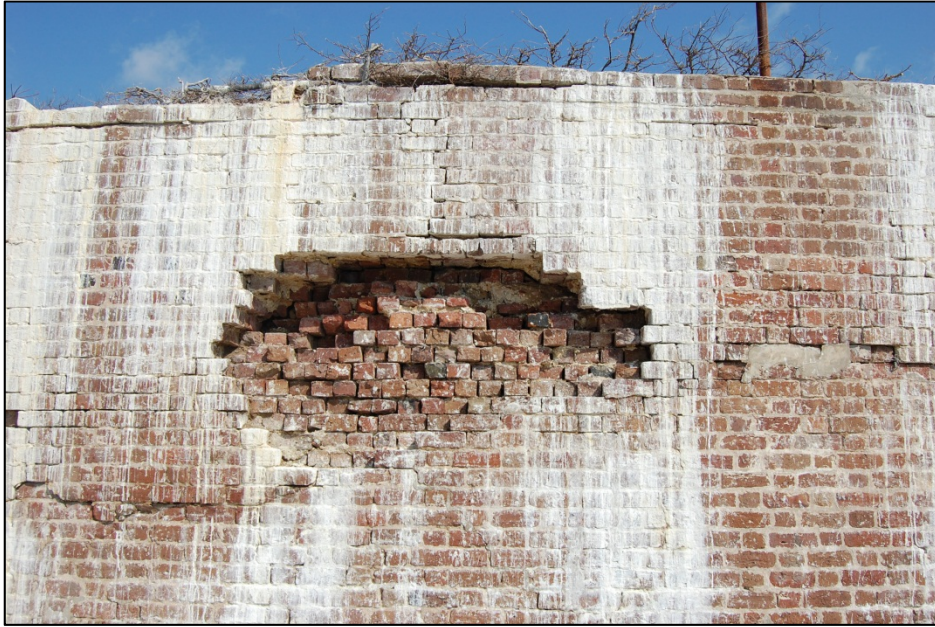
Figure 7.11 Showing missing brick patch. Damage caused by vegetation at top of wall is visible
