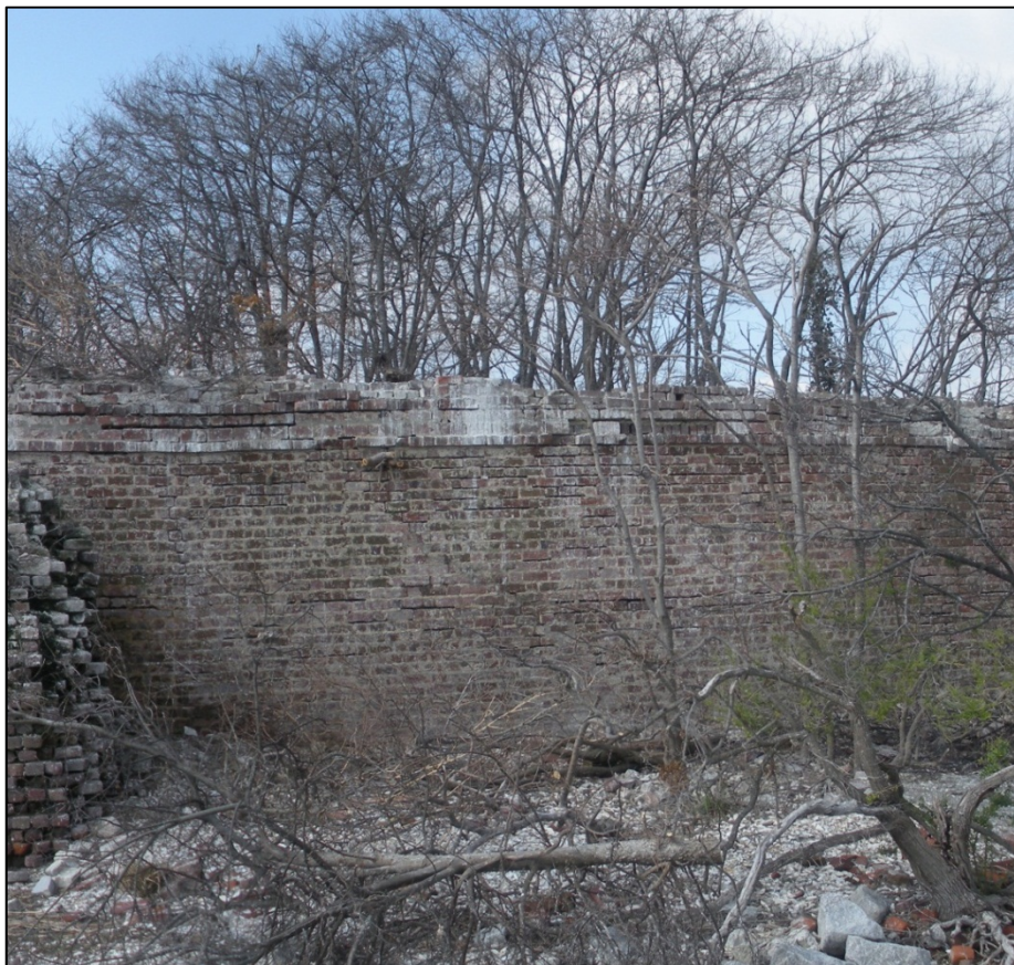
Figure 7.18 Showing extensive large tree growth and resultant deterioration of masonry at the top of the wall
