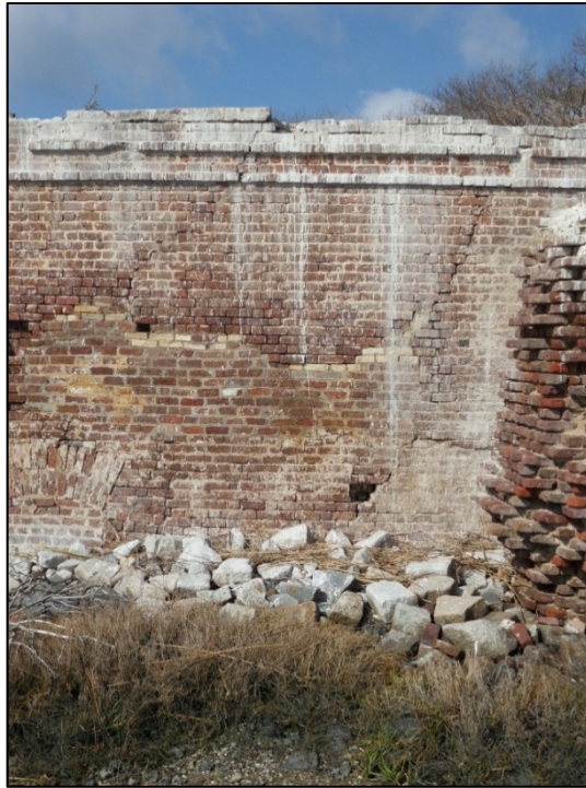
Figure 7.16 Showing Portland cement patch and adjacent diagonal fracturing
