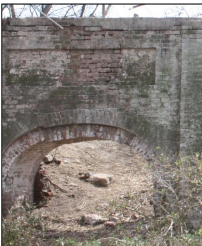
Figure 7.1: Detail above arch showing mortar joint decay and organic growth
