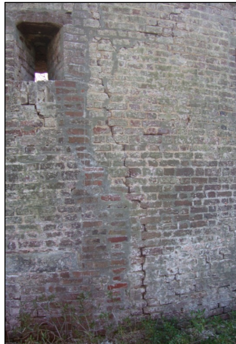
Figure 7.22 Showing fracture paralleling modern brick patch
