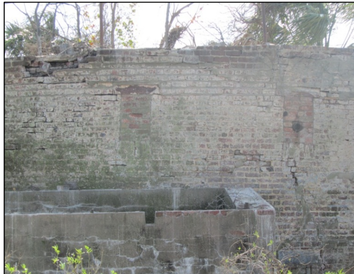
Figure 7.3 Major horizontal and diagonal fracturing and spalling brownstone header
