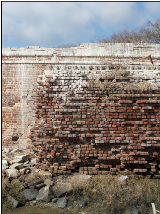
Figure 7.17 Showing unstable outer masonry wall
