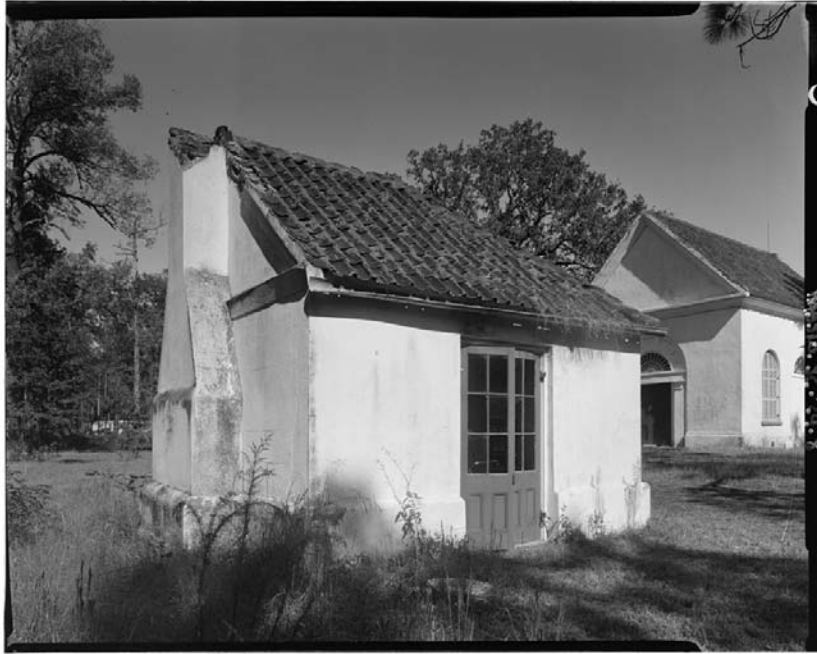
Figure 2.12. Vestry house with damaged chimney. Photo from Historic American Buildings Survey, Library of Congress, Prints and Photographs Division.
