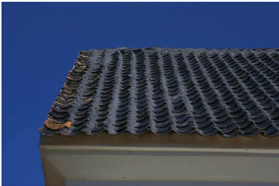
Figure 3.21. Pantiles coated in tar from 1937 restoration. Photo courtesy of 4SE Structural Engineers.
