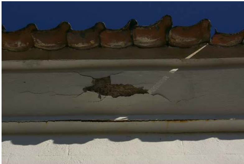
Figure 2.11. Exposed metal wire lath on southeastern cornice of church. Photo by author.
