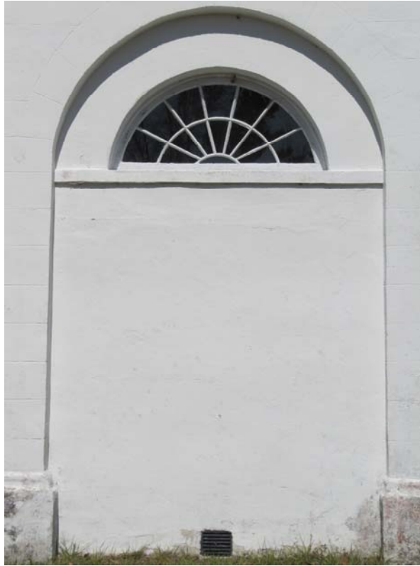
Figure 3.13. Photo depicting where former south doorway was blocked. Photo by author.
