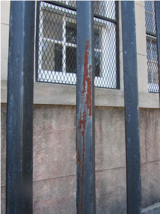
Figure B.6: Paint peeling.
