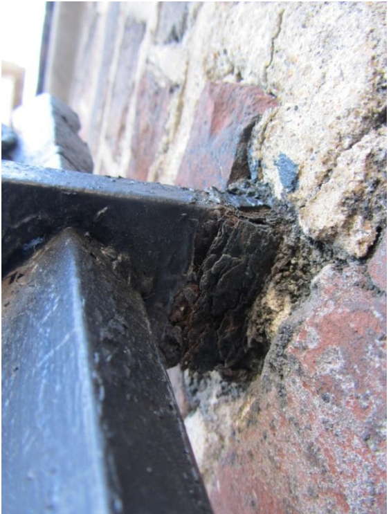
Figure B.7: Delamination.
