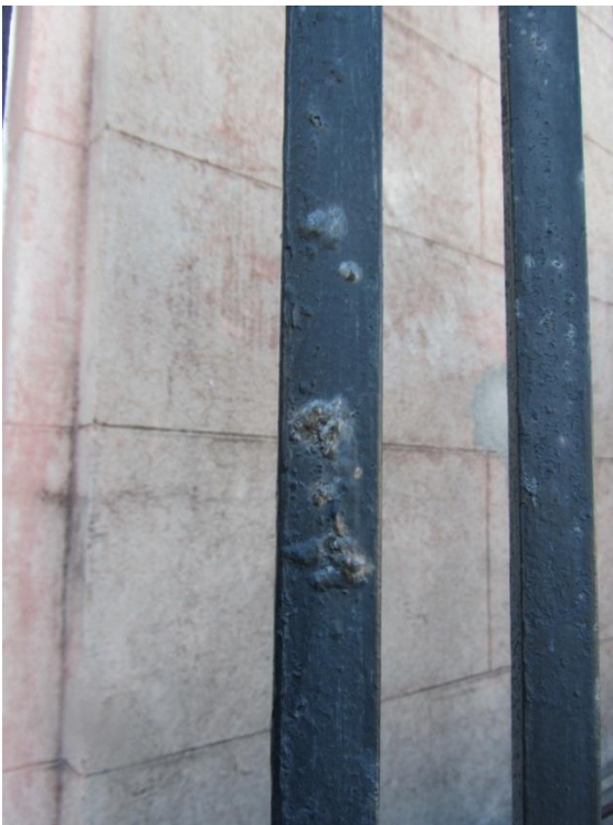
Figure B.2: Paint bubbles.
