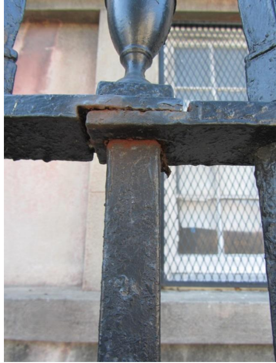
Figure B.5: Rust on connection point.
