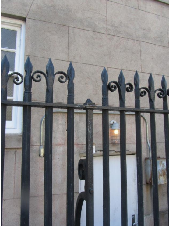
Figure B.4: Missing part.
