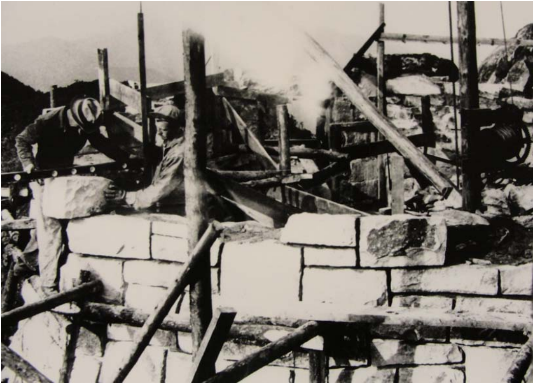
Figure 3.7: CCC men constructing fire tower in GRSM. Courtesy of GRSM Library, Mount Cammerer Fire Tower (White Rock) file, photo by Marshall Fox, 1936.
