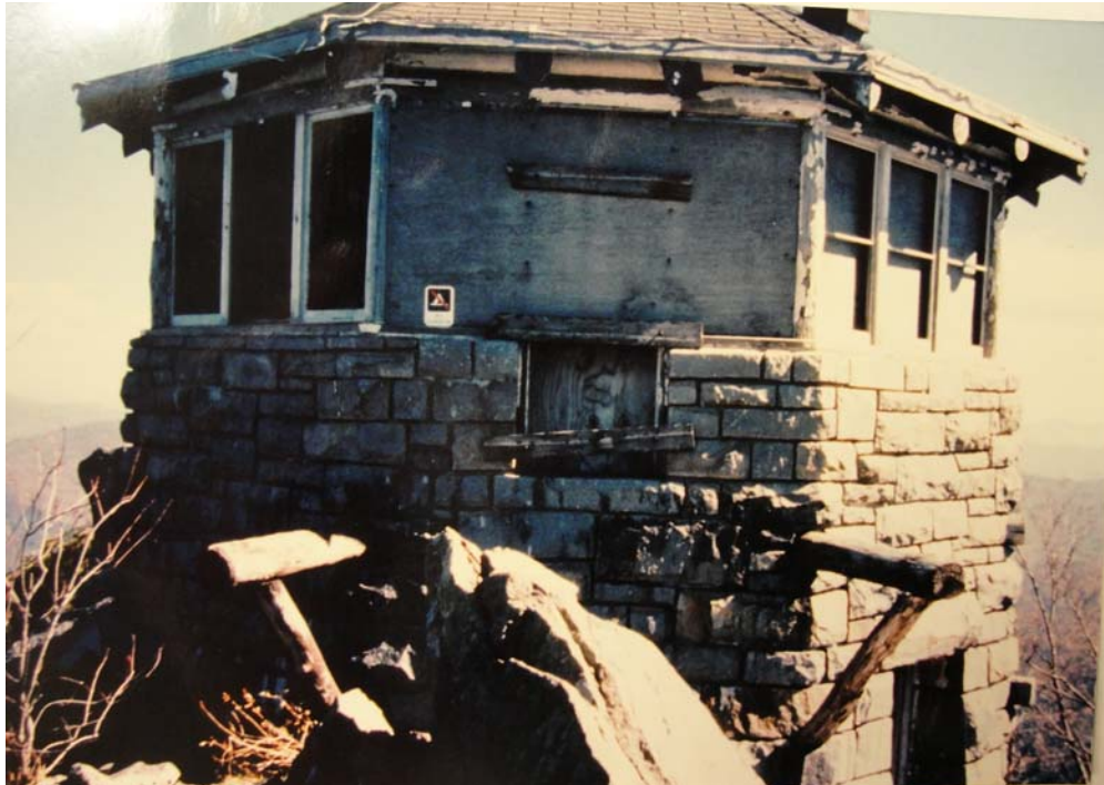
Figure 6.13: Mount Cammerer in state of disrepair, October 1989. Courtesy of GRSM Library.
