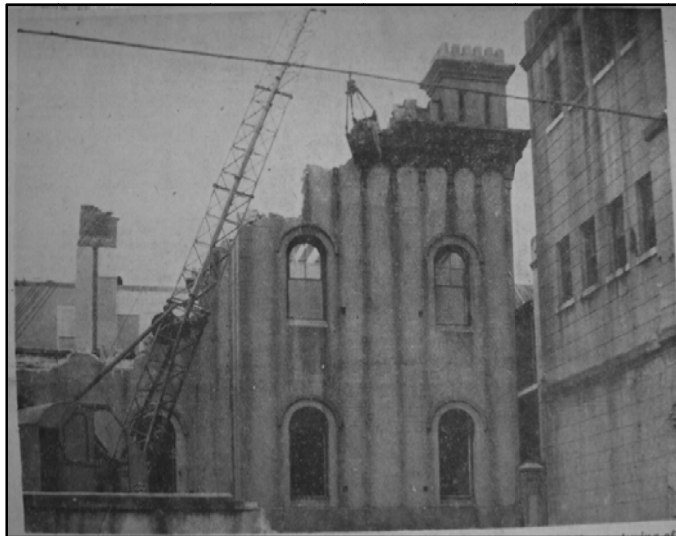
Figure 6.5 - Demolition of West Wing of Old Citadel in progress, News and Courier , "The Big Bite" January 28, 1958. Staff Photo.
