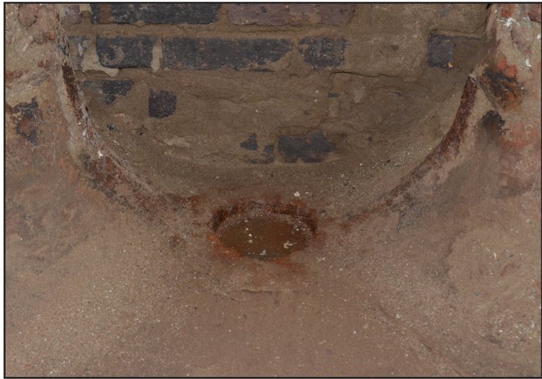
Figure 8.4: Filled cavity in pintle in casemate C-4. (photo by author)
