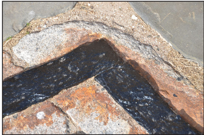
Figure 8.2: Traverse Rails along Left Face showing staining from pooling water. (photo by author)
