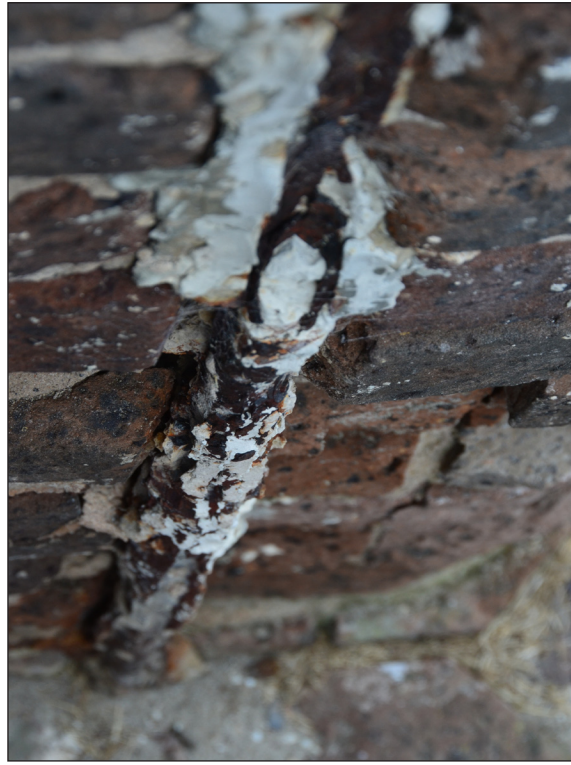
Figure 4.33 Detail of Gas Piping with multiple campaigns attempting to prevent water accumulation in the interior. Photo by author.
