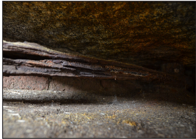
Figure 8.3: A-19 Pintle showing corrosion along slag lines. (photo by author)
