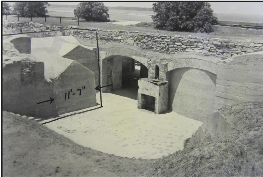
Figure 7.2 Left Flank fireplace in significantly better condition than the ruins found along the Gorge Wall (courtesy of Fort Sumter National Monument)
