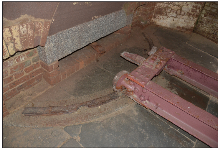
Figure 4.17 Traverse Rails inside Right Face casemate at Fort Sumter (photo by author)
