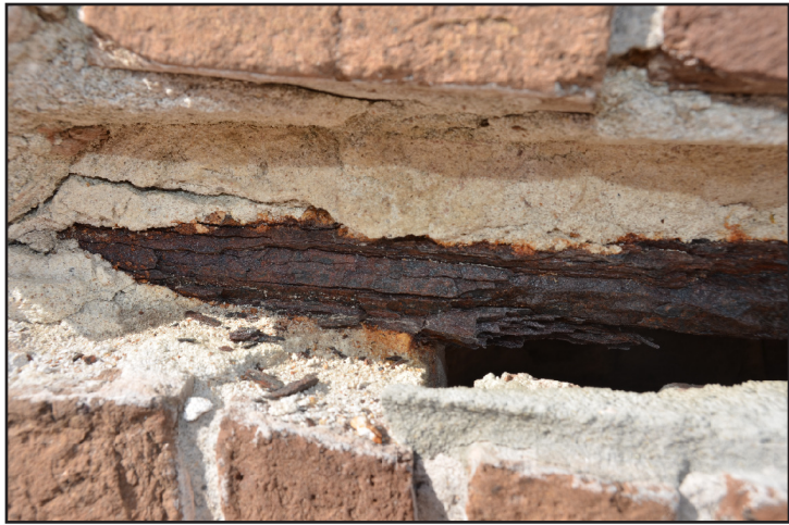
Figure 8.6 Mortar around emebbed tie-rod in Left Flank. (photo by author)
