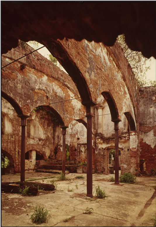
Figure 4.3: Sugar Mill in Puerto Rico utilizing combination of cast iron columns and masonry arches. (courtesy of the Library of Congress)
