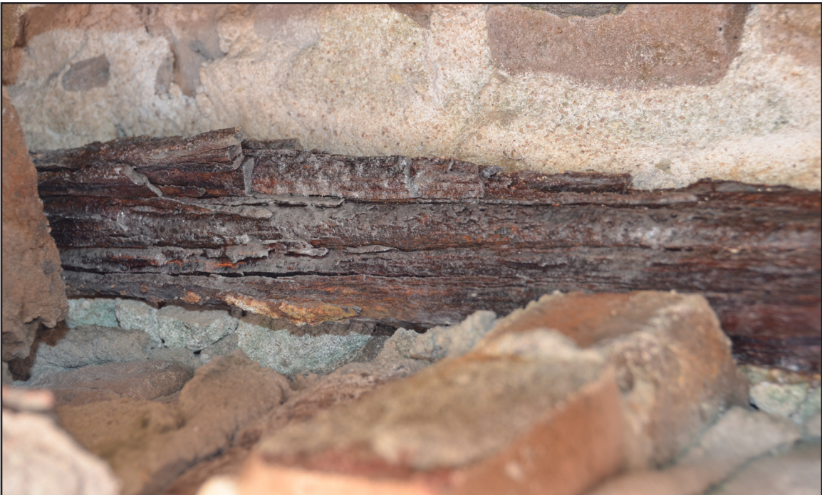
Figure 6.10 Interior detail of the Left Flank fireplace tie-rod showing remaining metal core and remaining corrosion. (photo by author)
