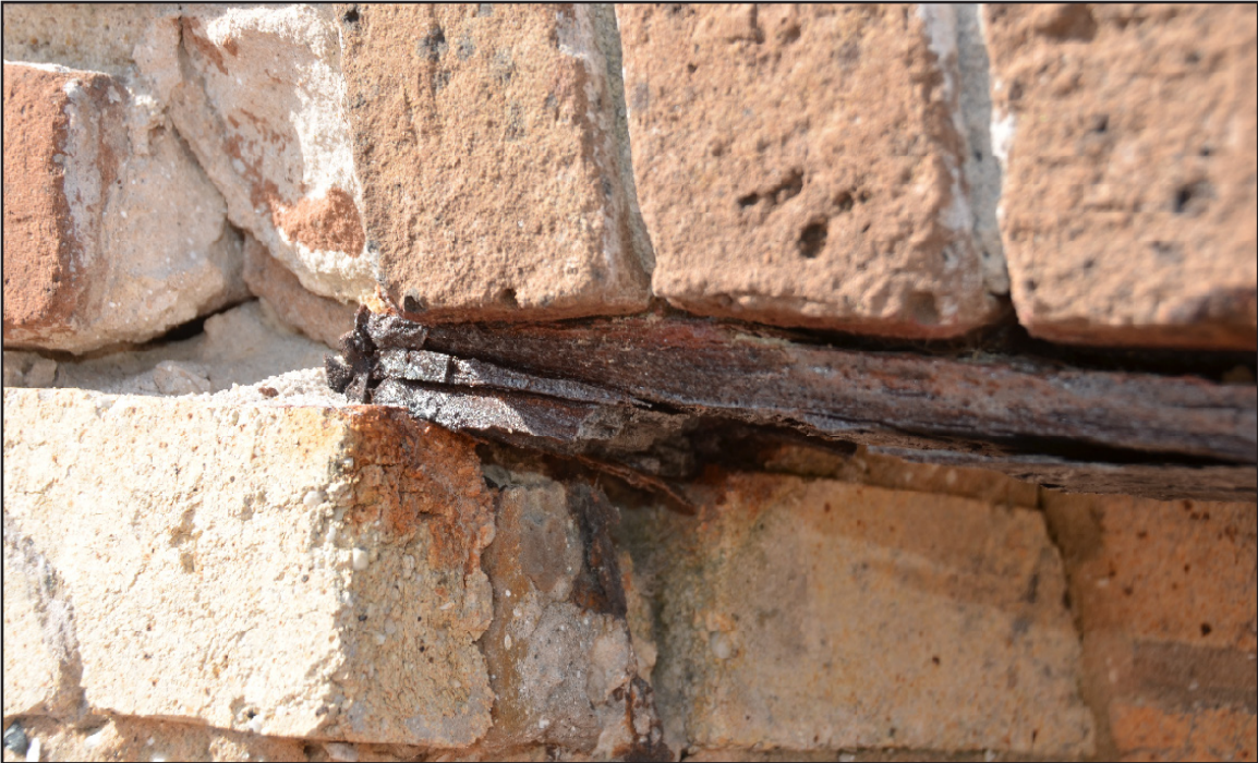
Figure 6.9 Detail of the Left Flank fireplace lintel showing remaining metal core and remaining corrosion after failure of lintel. (photo by author)
