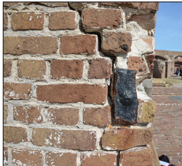
Figure 6.11 Cracking of the Left Flank fireplace due to the expansive corrosion of the tie-rod. (photo by author)
