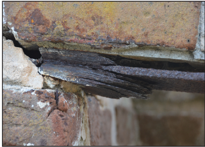
Figure 8.5 Metal loss in Gorge Wall fireplace lintel. Photo by author.
