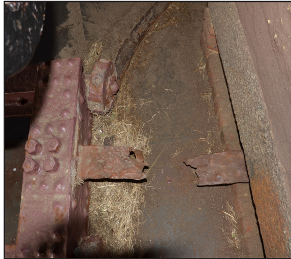
Figure 4.22: Image detailing corroded and broken pintle from Right Casemate (photo by author).
