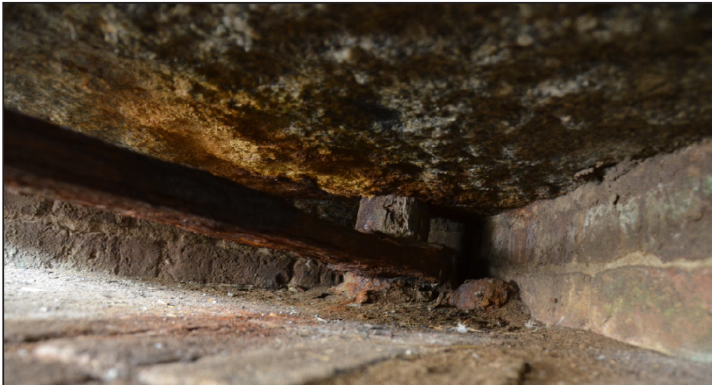
(top) Figure 6.13 Brick rubble cement around pintle in Left Flank embrasure. (photo by author)
