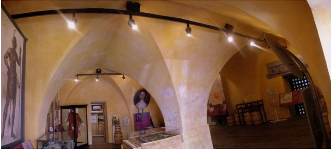
Figure 4.3: Interior panorama showing the iron tie rods exposed in the powder magazine ceiling vault. (Photo taken by author)
