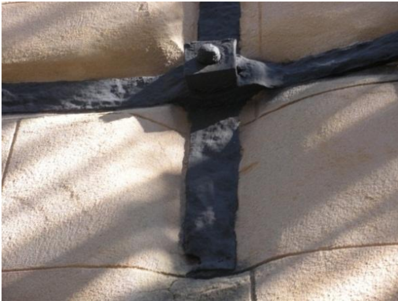
Figure 5.3: South-west anchor plate showing severe deterioration. (Photo taken by author)
