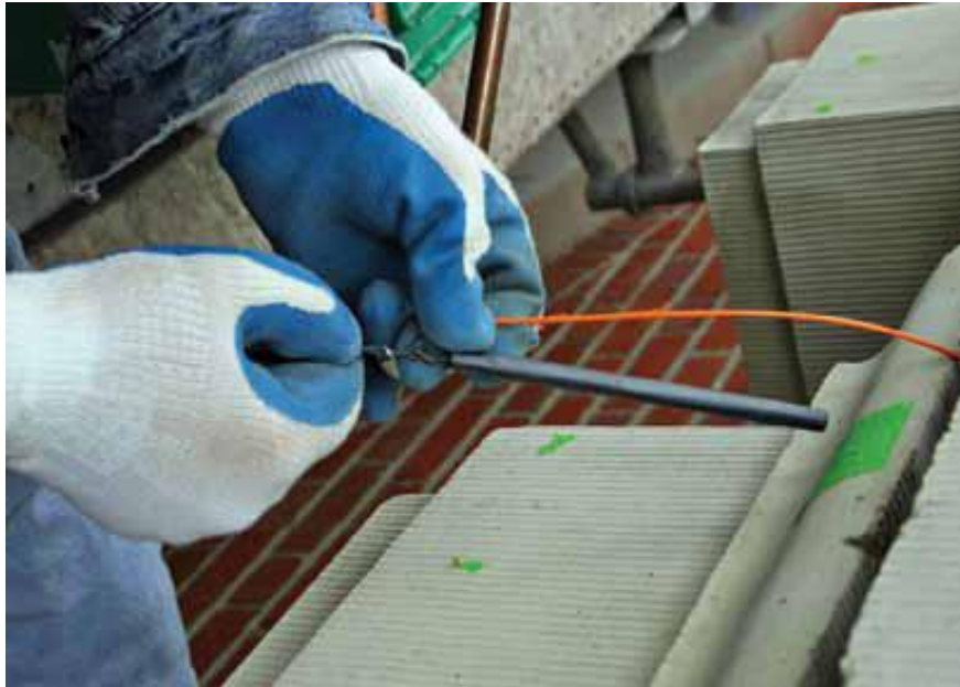
Figure 5.9: Discrete anode connected to power supply and ready for placement into mortar joint. (Source: Kelly Page, ed., "Cathodic Protection of Historic Terra Cotta Cornice", Concrete Repair Bulletin (May/June 2009): 20-23, accessed 27 January 2012, www.icri.org )
