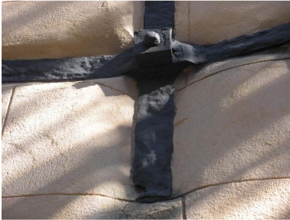
Figure 4.5: Close up photograph of the anchor plate on the south-west gable showing extreme deterioration. (Photo taken by author)
