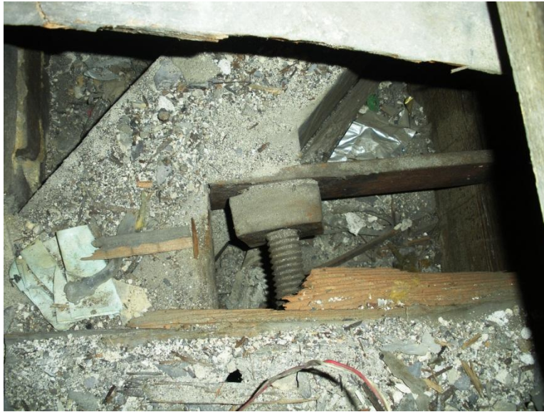
Figure 4.17: Tie rods installed in 1811 are threaded at their ends and secured to diagonal roof beams with bolts. (Photo taken by author)
