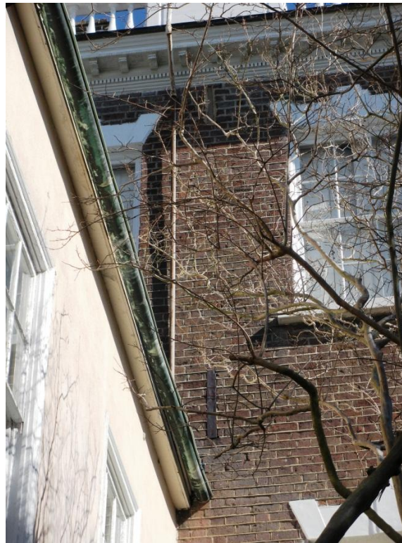
Figure 4.15: Vertical Iron straps indicate the insertion of tie rods on the rear wall of the main house following the 1811 tornado. Masonry damage just below the cornice indicates the placement of additional tie rods between the third floor and attic. ( Photo taken by author )
