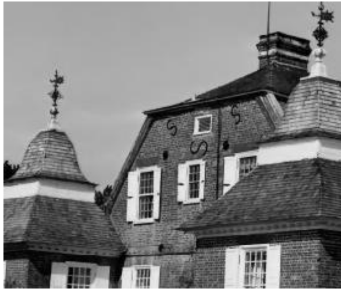
Figure 2.9: 'S' type wall anchor plates at Mulberry Plantation (1714), Berkeley County, SC (Source: "Mulberry Plantation, Berkeley County SC", National Register Properties in South Carolina, http://www.nationalregister.sc.gov ).
