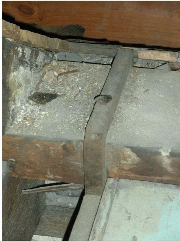
Figure 4.29: End attachment detail of the tie rod where the rectangular rod clamps over the sill plate within the roof structure. (Source: Photo taken by author)
