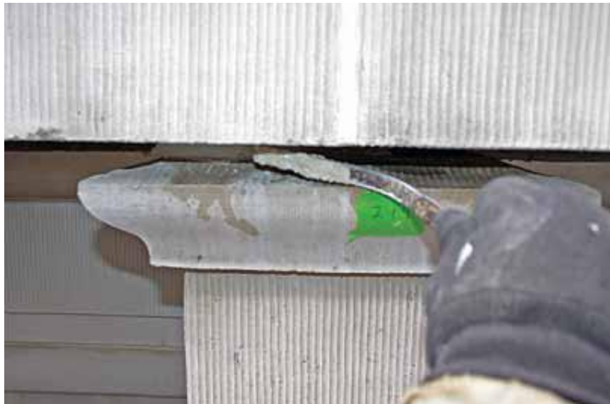
Figure 5.10: Placement of lime-based mortar after anode and reference electrode installation. (Source: Kelly Page, ed., "Cathodic Protection of Historic Terra Cotta Cornice", Concrete Repair Bulletin (May/June 2009): 20-23, accessed 27 January 2012, www.icri.org )
