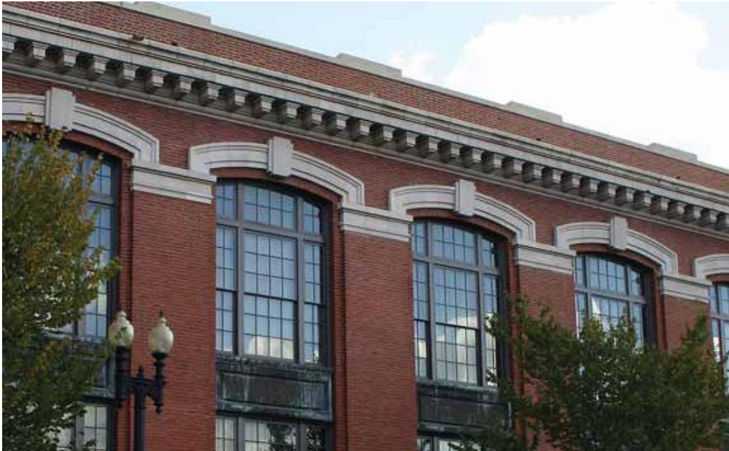
Figure 5.8: A view of the restored terra cotta cornice at the National Holocaust Museum in Washington, D.C. (Source: Kelly Page, ed., “Cathodic Protection of Historic Terra Cotta Cornice”, Concrete Repair Bulletin (May/June 2009): 20-23, accessed 27 January 2012, www.icri.org )
