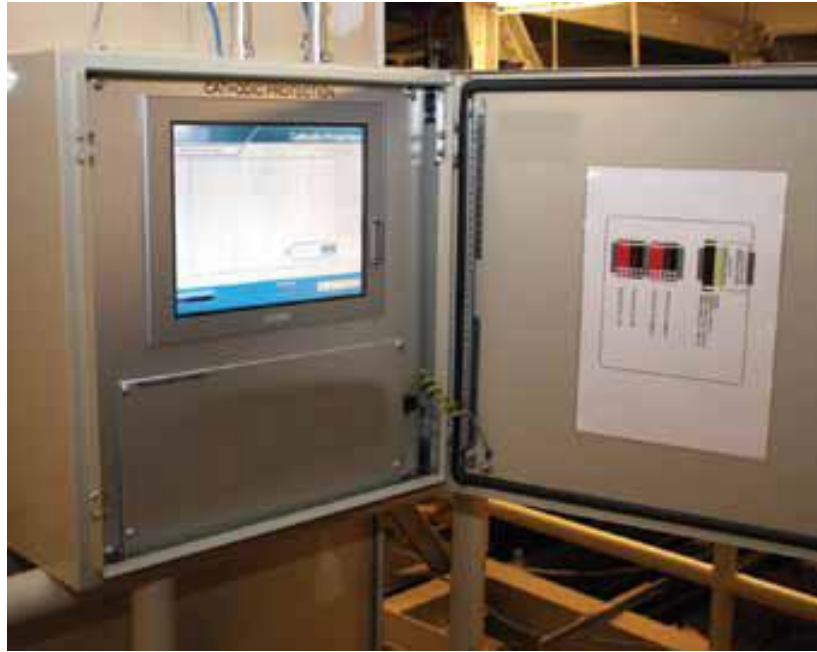
Figure 5.11: Monitoring equipment installed inside the building allows for remote monitoring and system adjustment. (Source: Kelly Page, ed., “Cathodic Protection of Historic Terra Cotta Cornice”, Concrete Repair Bulletin (May/June 2009): 20-23, accessed 27 January 2012, www.icri.org )
