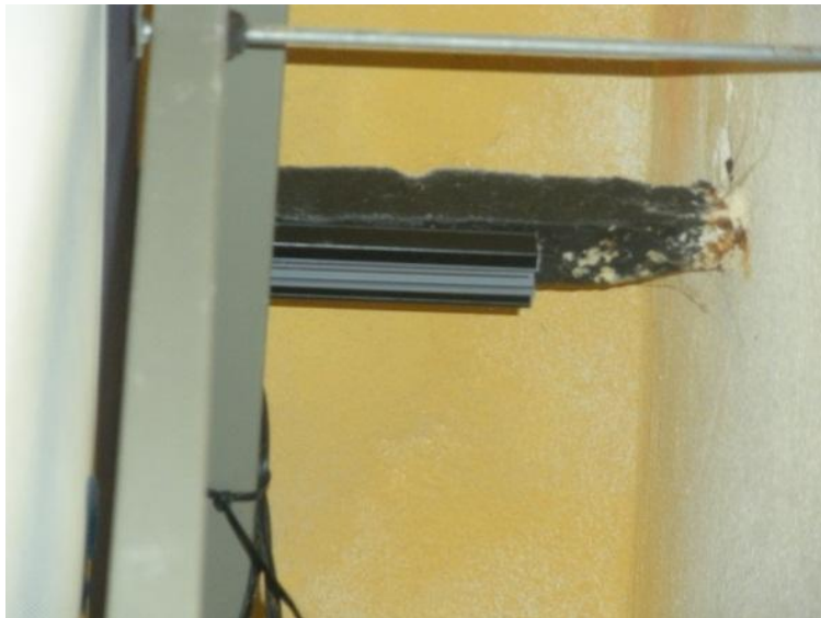
Figure 5.1: Localized corrosion where rectangular tie rod enters interior wall. (Photo taken by author)
