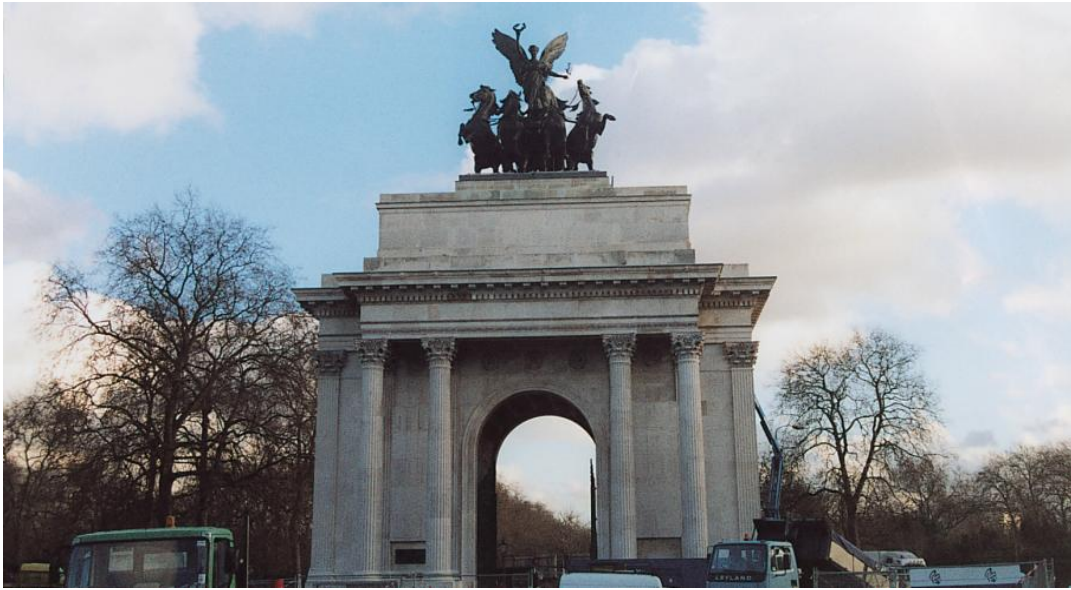
Figure 5.6: The Wellington Arch, Hyde Park, London; constructed in 1820, a recent inspection revealed significant corrosion of the steel I-beam supporting the Quadriga sculpture. (Source: Farrell and Davies. "Cathodic Protection of Iron and Steel in Heritage Buildings in the United Kingdom". APT Bulletin 36, 2005)
