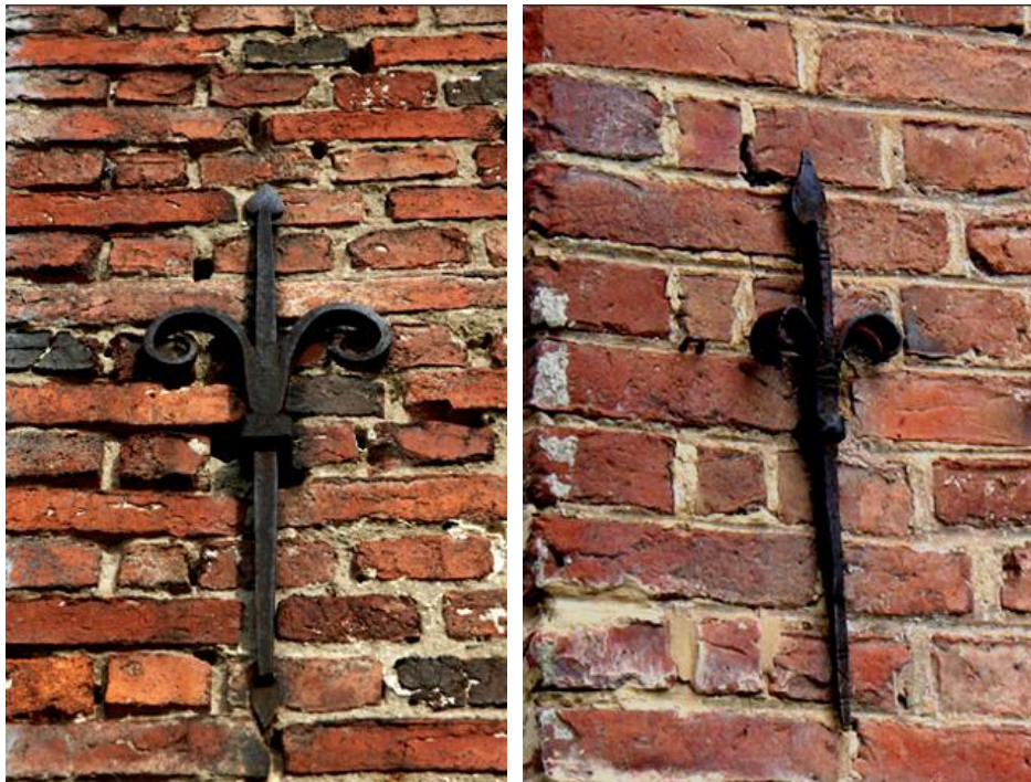
Figure 2.7: Dutch inspired wall anchors: Left: Van Hoesen House (1740) & Right: Pieter Winne House (1720). (Source: Van Hoesen House Historical Commission , http://www.vanhoesenhouse.org )
