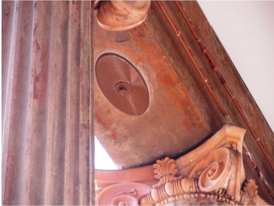
Figure 4.38: Photo showing the brownstone entablature and underneath the portico roof. The oval pattern plates can be seen securing the brownstone entablature with the tie rod and turnbuckle tying the portico side walls behind the entablature. (Photo taken by author)
