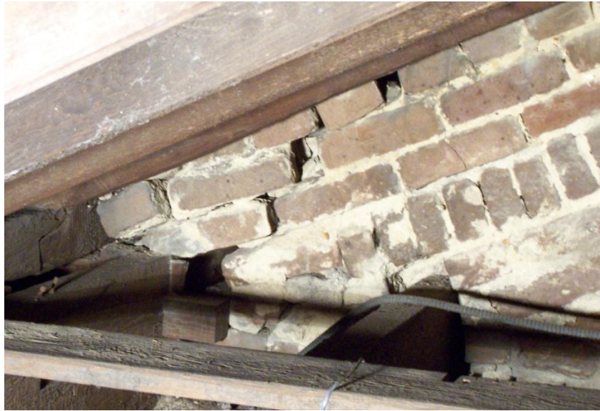
Figure 4.35: Portions of the brick portico gable at Randolph Hall , originally damaged in the 1886 earthquake, showing signs of additional movement. (Photograph provided by 4SE, Inc.)
