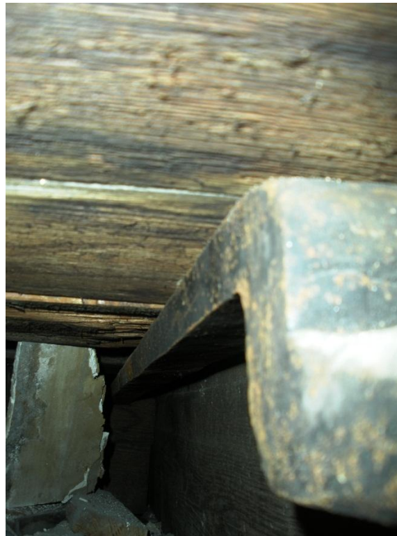
Figure 4.16: An 1811 tie rod installed to correct tornado damage projects through the attic floor in between joists. (Photo taken by author)
