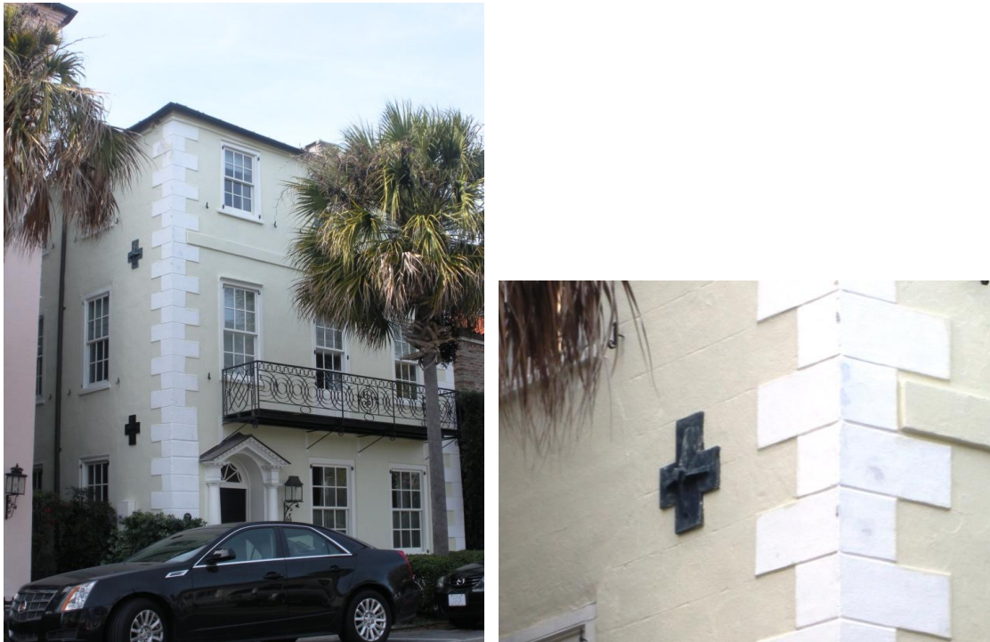
Figure 4.23: Left: Cruciform shaped anchor plates installed at 57 East Bay Street; Top: Anchor plate detail ( Photos taken by author )
