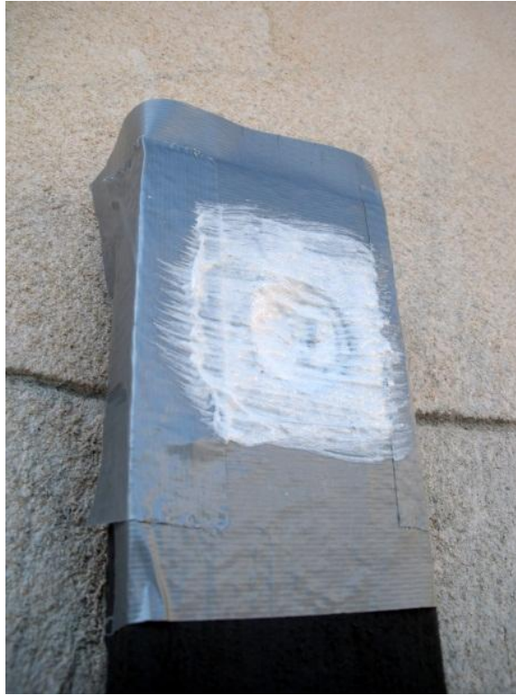
Figure 4.10: After initial cleaning and brushing, a layer of Smart Strip is applied to the area to remove top layers of paint. (Photo taken by author)
