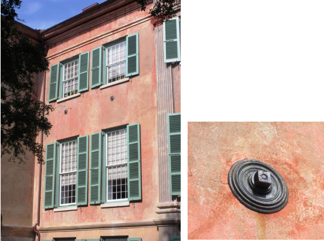
Figure 4.33: South wall of the Main Building, east of the portico showing two earthquake bolts installed between the first and second floors. Detail: Circular patterned plate with decorative, moulded profile. (Photos taken by author)
