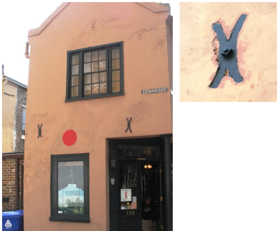
Figure 2.10: An early 'butterfly'-shaped wall anchor on an 18 th century structure at 91 Exchange Street, Charleston, SC (Photos taken by author)
