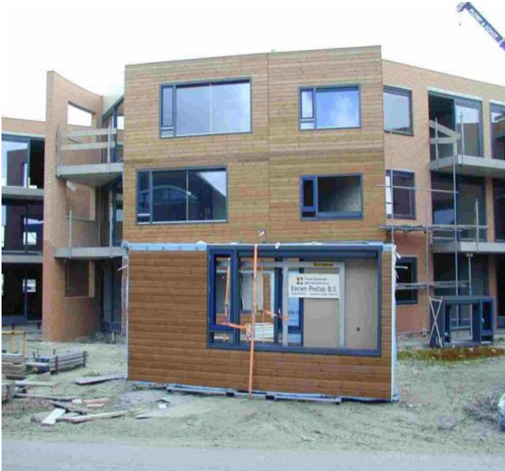
Figure 2.3 Panelized wall with cladding, interior and exterior finishing (Courtesy of Pulte Home Sciences)
