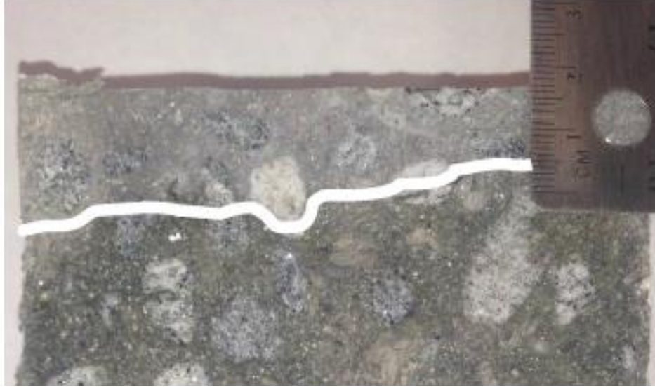
Figure B.3. Chloride penetration after three month
