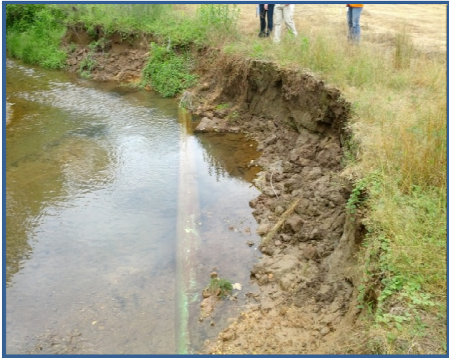
Figure 1. Exposed gas line prior to project implementation.
