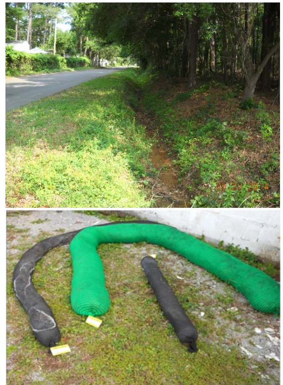
Figure 1. Bacteria media filter strips and one of several target sites along roadside ditches.
